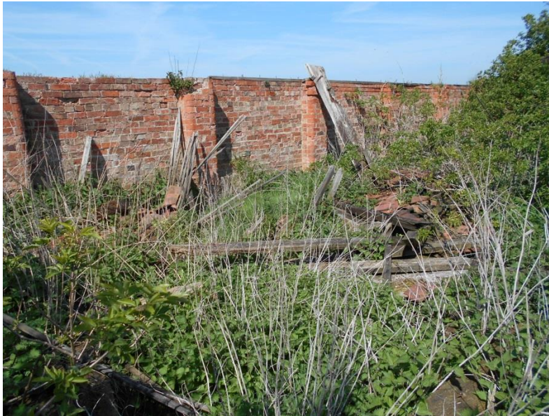
Fig 17: The ruined Building 11, its roof collapsed in
