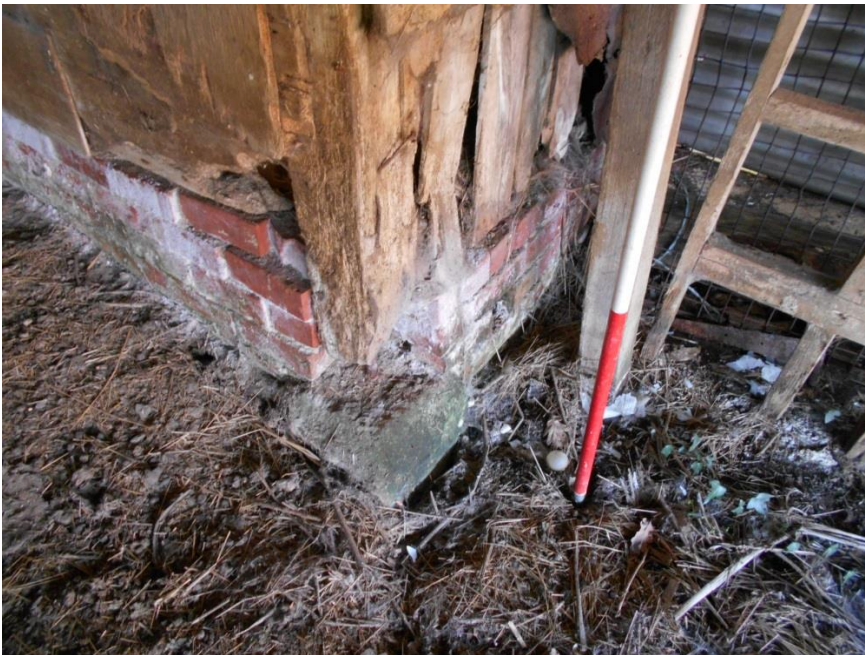
Fig 6: Original front chamfered plinth block on which rested the former open front of Building 2; scale 1m
