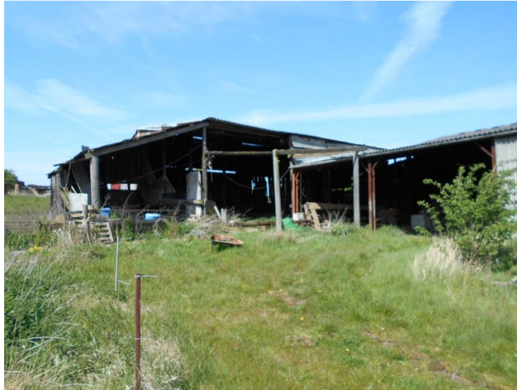
Fig 15: Building 9 looking west, Building 10 to right. At far left in the distance is the ruin Building 11.
