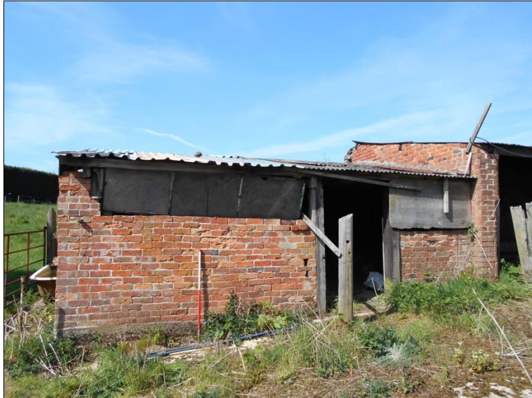
Fig 10: The southern half of Building 5, looking west; scale 1m; the footpath can be seen on top of the rise at far left
