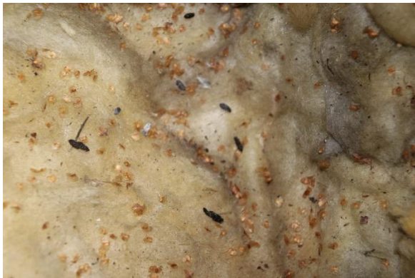
13. Scattered bat droppings on insulation
