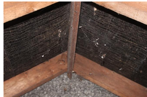
16. Cobwebs in ridge in most buildings
