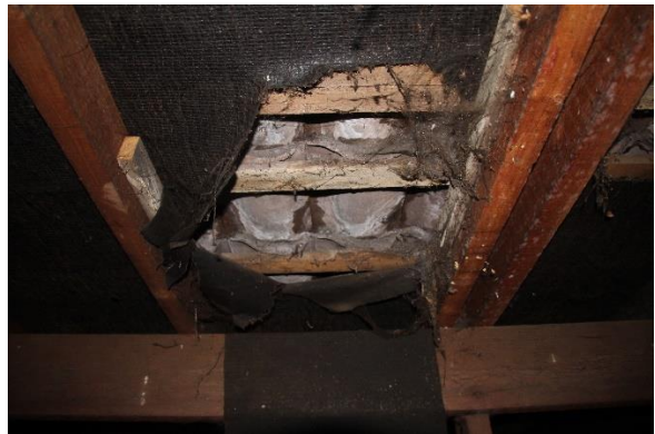
12. Cob-webbed gap showing tightly fitting tiles
