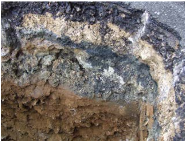
Photo 14 (left) showing trial pit 238, with horizon of visually hydrocarbon impacted material
