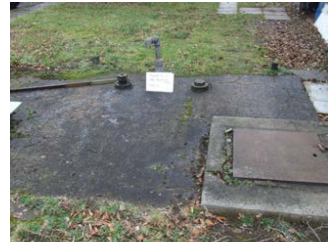
Photo 10 (right) showing tanks UGNSA 34 and 35.
