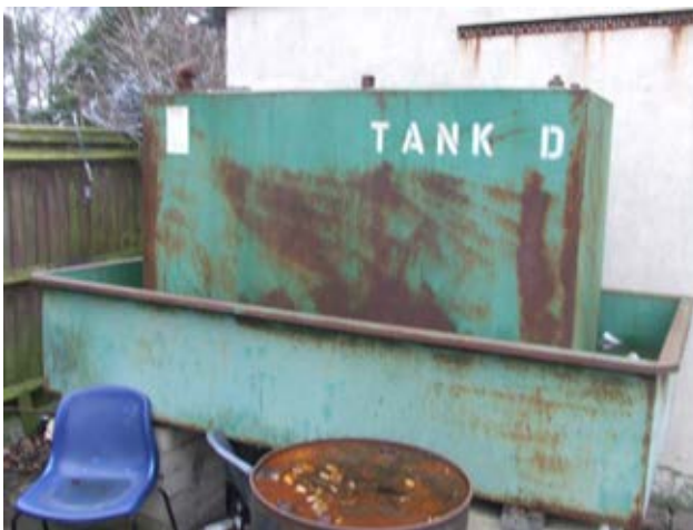
Photo 4 (left) showing tank AGNSA 08
