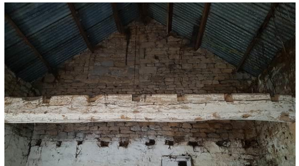
33. Gaps in internal barn walls
