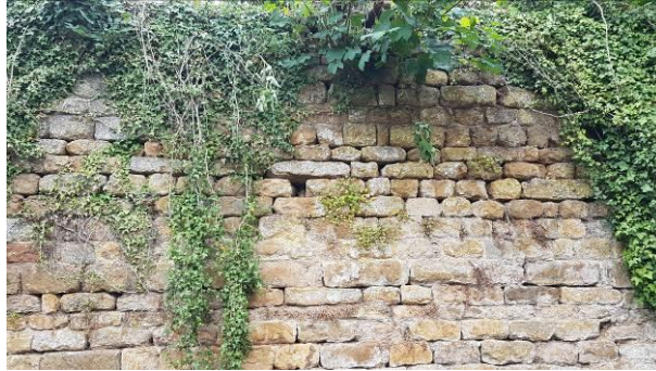
37. Gaps in stone wall
