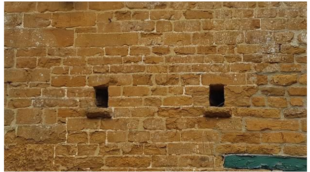
29. Gaps in wall
