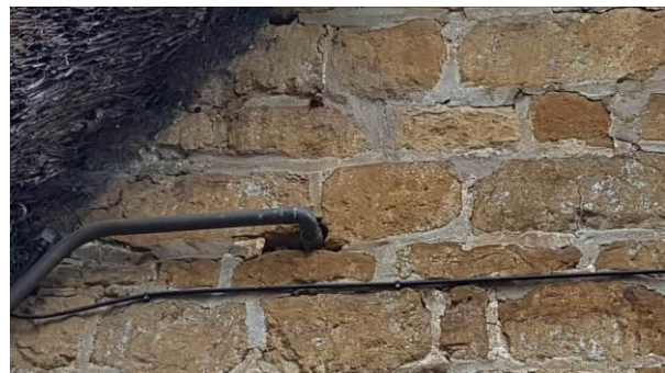
12. Gap around pipe work
