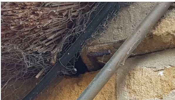
11. Gap at top of wall under thatch
