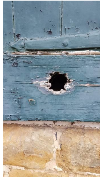
14. Hole in boarded door
