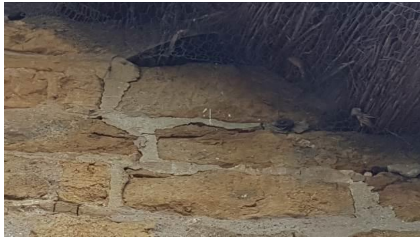
10. Gap at top of wall under thatch
