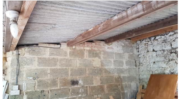
31. Gap at top of wall
