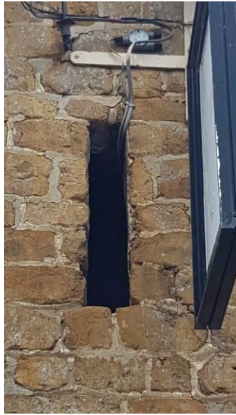
13. Hole in wall
