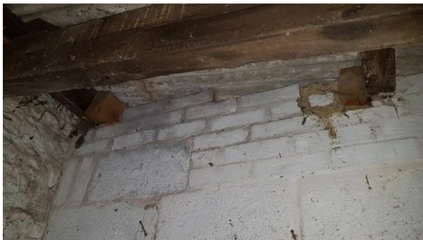
32. Gap between joists and boarded roof
