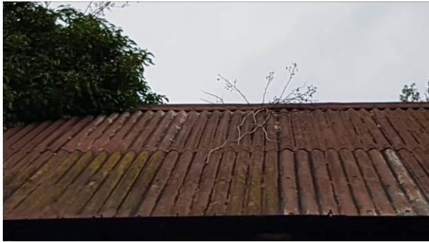
28. Gaps under roof overlap
