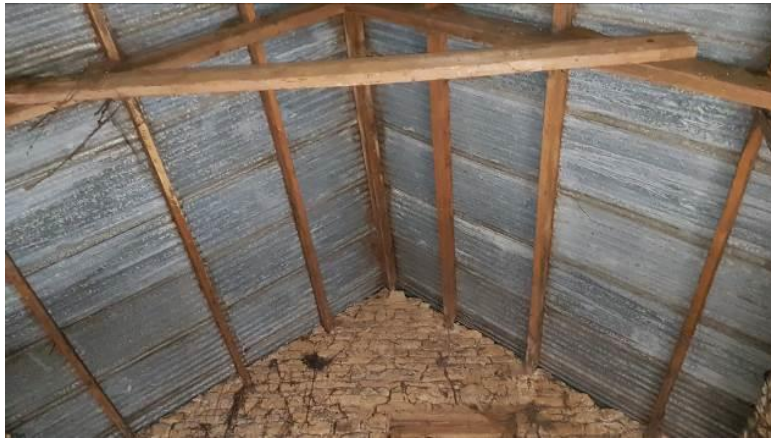
34. Gaps between joists and tin roof
