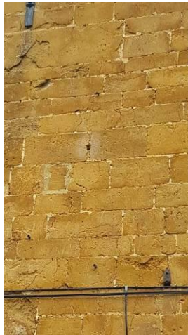
9. Gaps in stonework
