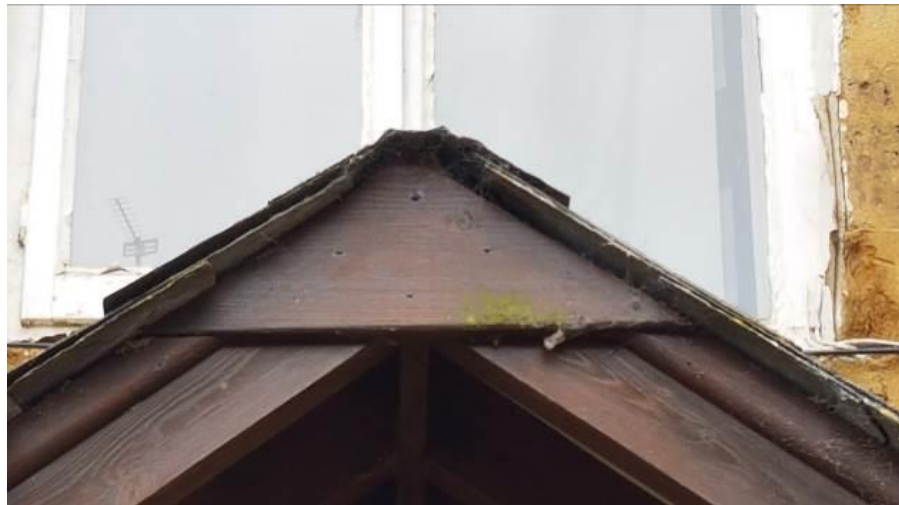
16. Gaps under slates
