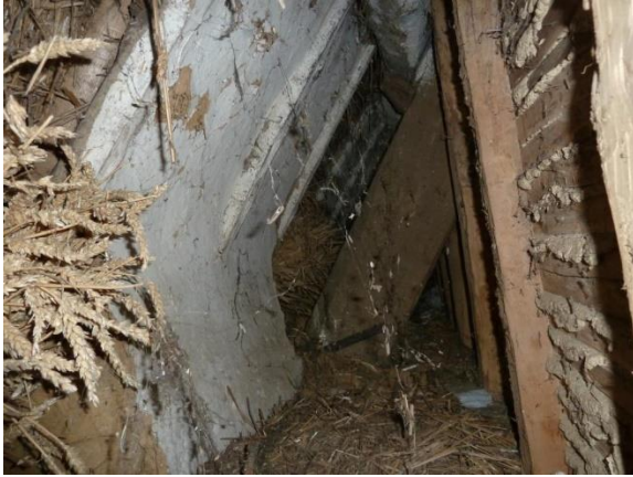
In the side North wall in Room M is a low access door to view eaves. View East with Cruck
