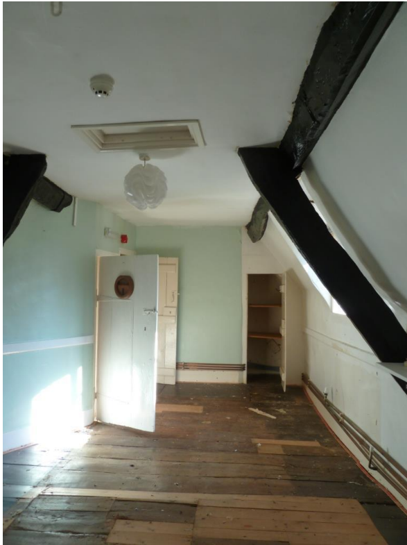
View East Room L . Cruck Truss The Second floor over the main building extends over Rooms I & J below.
