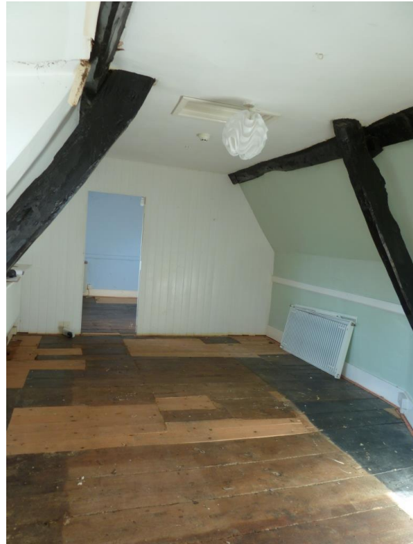
View West Room L Cruck Truss The Second floor over the main building extends over Rooms I & J below. Dividing Wall to Room M
