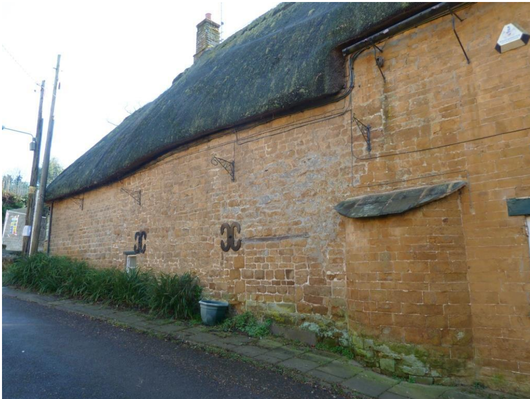
Stone half circular built bread oven with a C20 slate covering; Stone wall has X2 Iron wall anchor plates. Evidence in GF of a previous door opening with timber lintel and evidence of possible former window opening central FF
