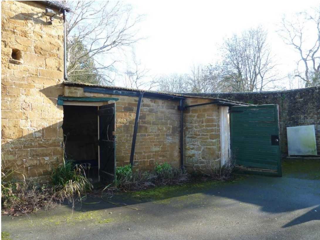
To south side of Stable are x2 a single storey stone outbuildings
