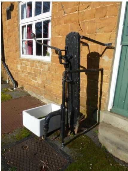
Hand water pump outside central door that is blocked from inside.
