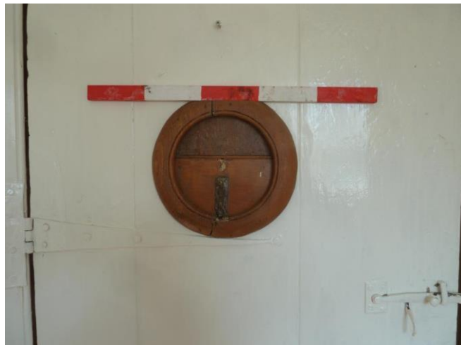
Portal/peephole in Main door with unusual unpainted circular timber sliding surround. 50cm scale
