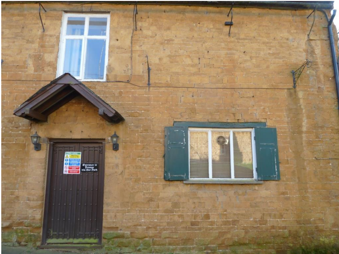
Central early C19 door entrance with dressed stone lintel with keystone, window with timber lintel and likely early C19 shutters
