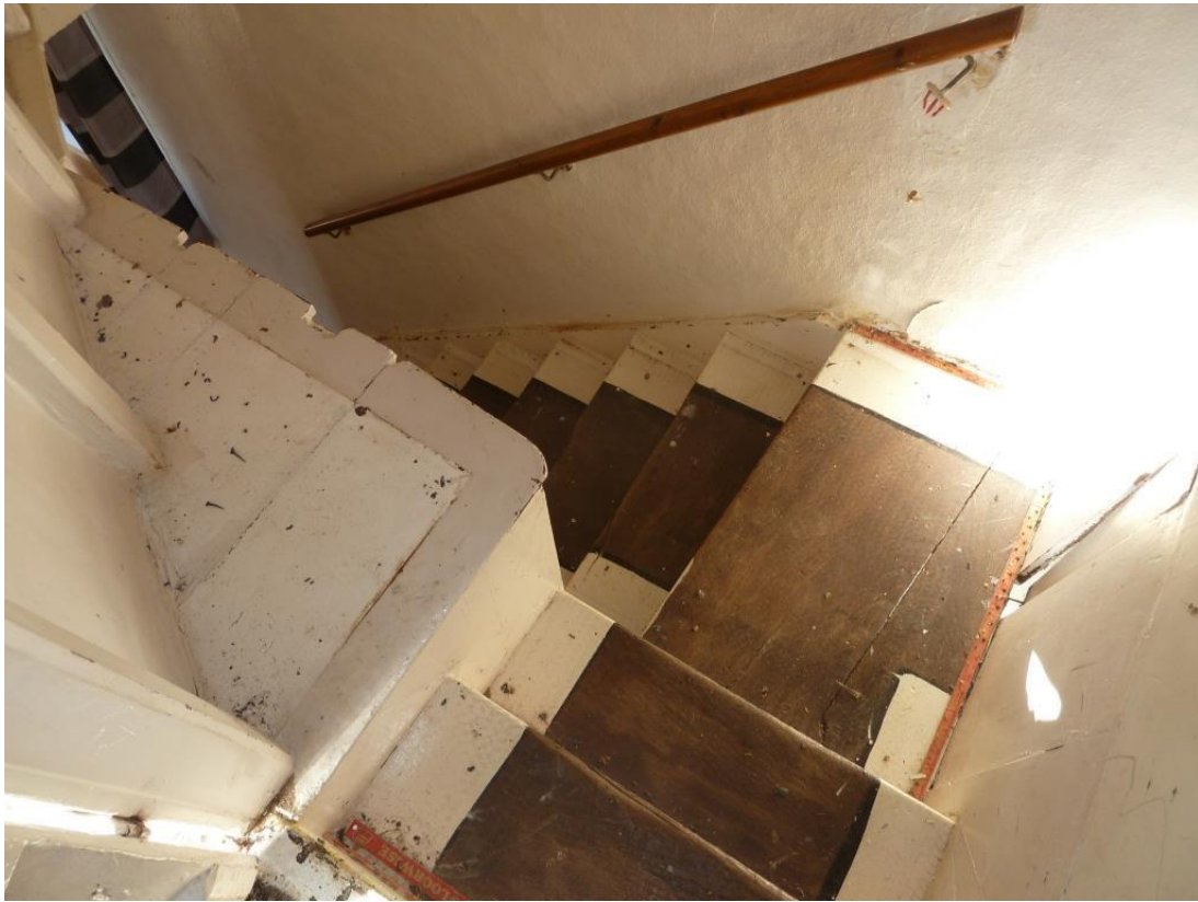
Attic Room/s are approached by a staircase K in the North elevation wall
