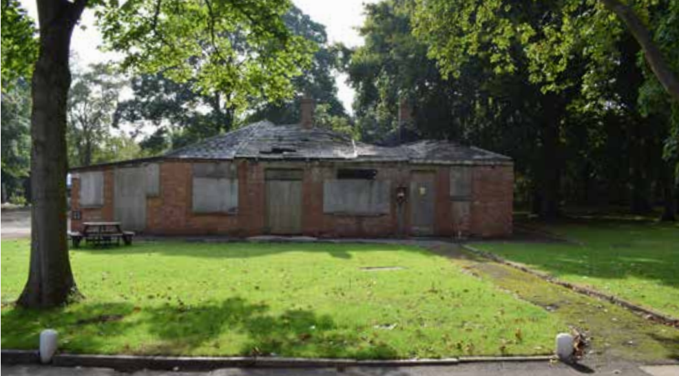
Fig 23: Building 144, currently in poor condition
