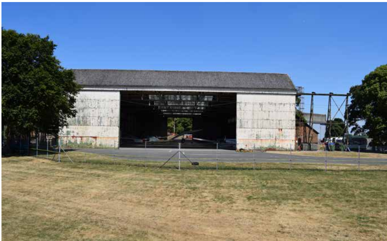
Fig 30: Type A Hangar with sliding doors in each end of the building
