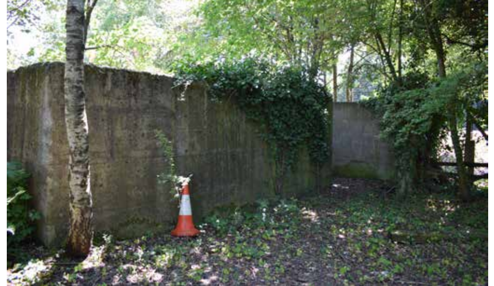
Fig 29: Sandwiched amongst the overgrown scrub between the old lane and new Skimmingdish Lane is a concrete walled compound, thought to have been a former pyrotechnics store area.
