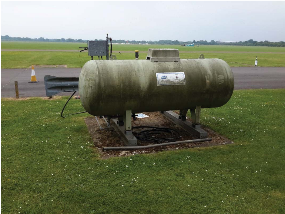
Plate 7 Liquefied Petroleum Gas Storage Tank
