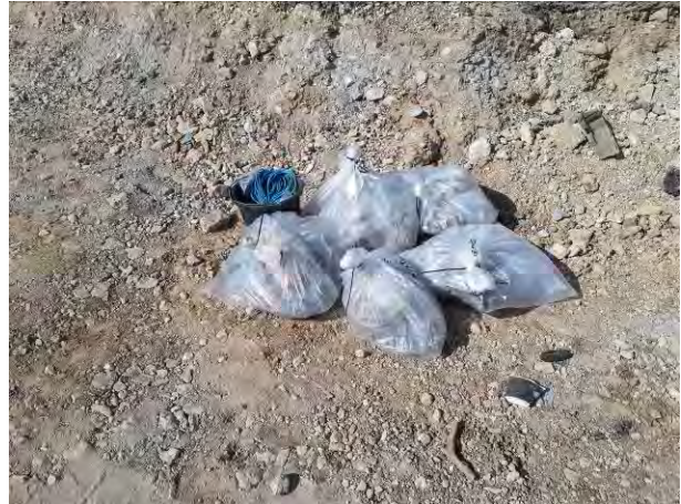
21.06.18 – Handpicked ACM cement sheeting double-bagged, zip tied and then removed offsite for disposal.
