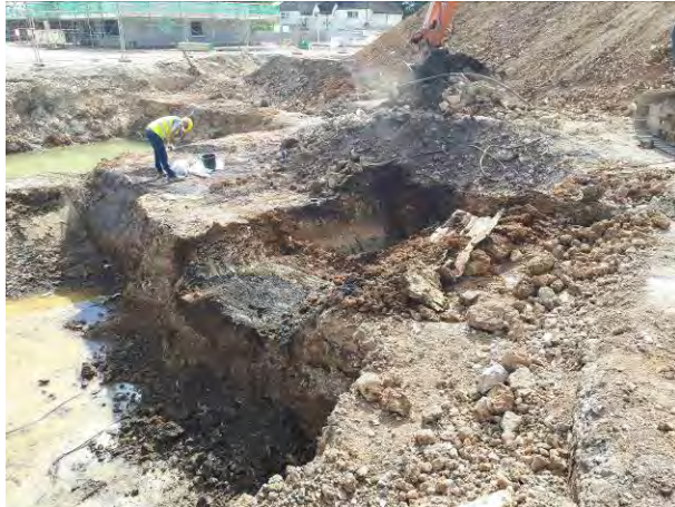
21.06.18 – Handpicking of visible ACM cement sheeting and excavation of surrounding soils for removal to quarantine area.
