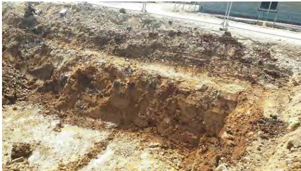
28.06.18 - View of western end of southern sidewall; no significant contamination indicators observed.
