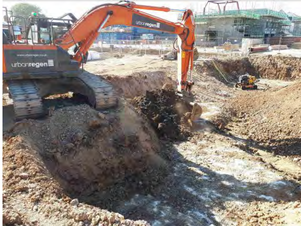
02.07.18 - Continued excavation of hydrocarbon contaminated soils down to weathered bedrock in northeast corner.
