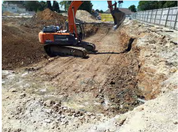
02.07.18 – View along northern extent of excavation; residual staining present on eastern part of sidewall.
