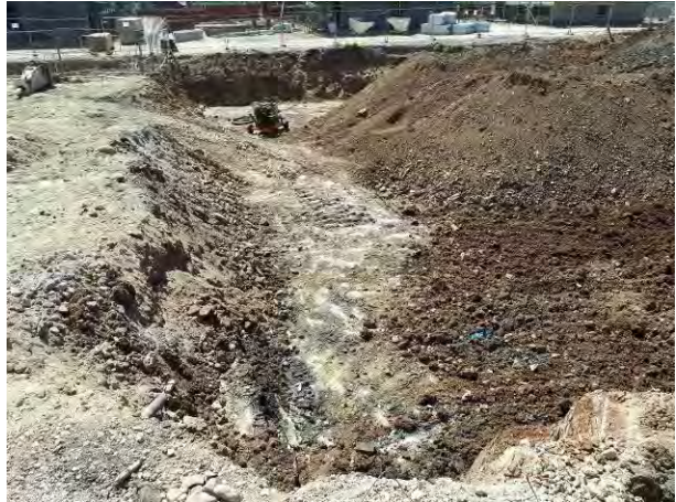
02.07.18 - View along eastern extent of excavation comprising weathered bedrock with some residual staining.
