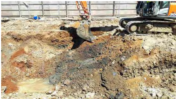
29.06.18 - Continuation of excavation down to natural bedrock along central part of northern extent; contamination encountered and removed.
