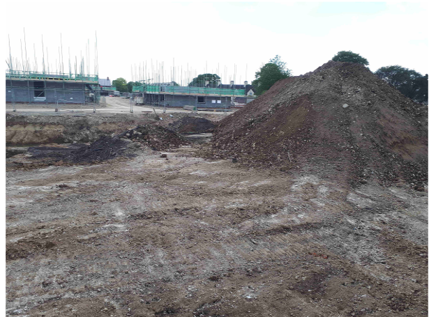
21.06.18 - Stockpile of recovered soils retained for replacement moved to west of excavation.
