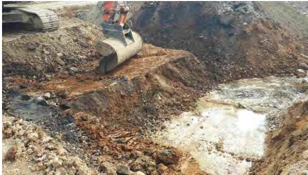
28.06.18 – Continuation of excavation down to natural bedrock along western extent; no significant contamination indicators observed - soils sampled and retained.
