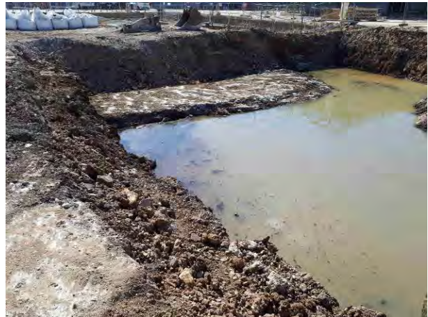
22.06.18 – Black floating product observed on pooled water within excavation.
