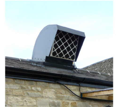
Close-up of extractors
