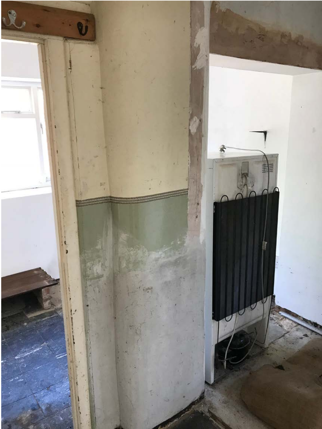
Openings to be in filled to create new Play room (note: in fill will not obscure existing piers)
