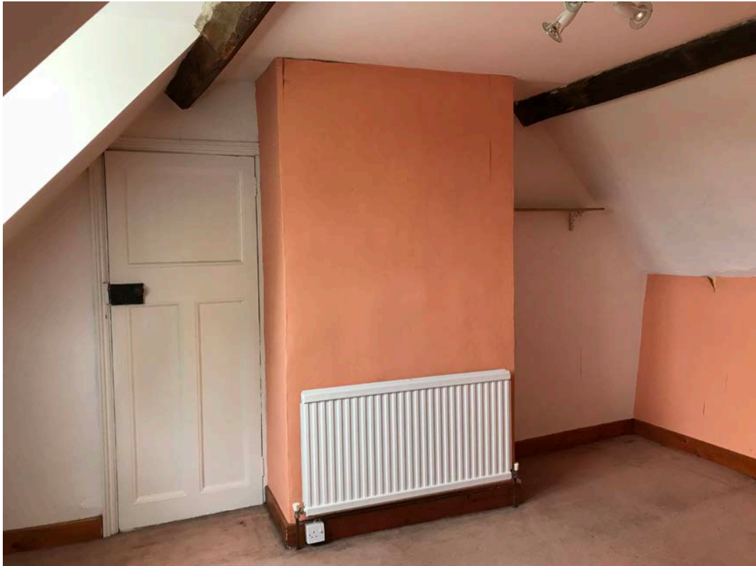
Ceiling to be removed and vaulted as per reciprocal bedroom at second floor
