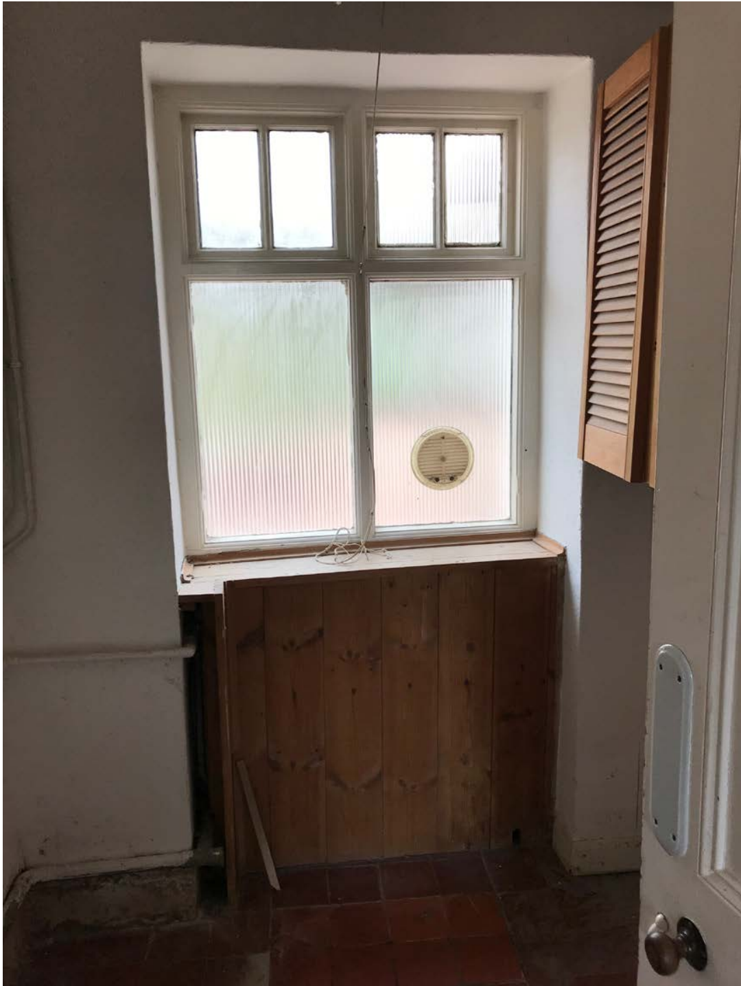
Internal view of existing window to be replaced by door way from hall to garden room
