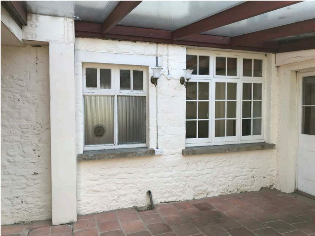
Smaller window to be replaced with new door way onto Hall. Note: Soil pipe moved to new location hidden within new WC
