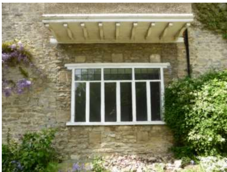
Figure 9: Modified ground floor window and evidence for straight joints to the left and right
