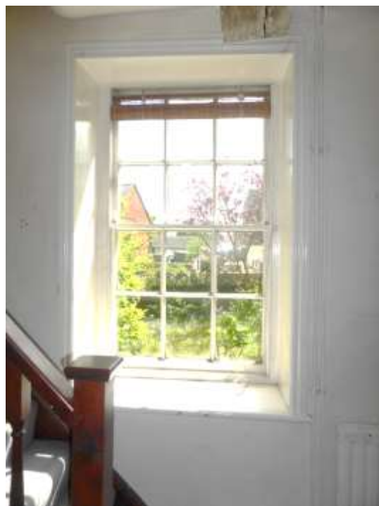
Figure 23: Six over six sash window in G1 with chamfered glazing bars and later 19 th century style fastener
