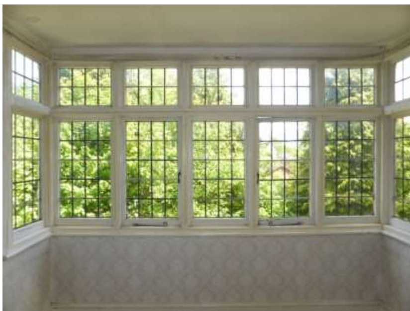
Figure 53: Detail of the early 20 th century leaded lights to the oriel window in F5
