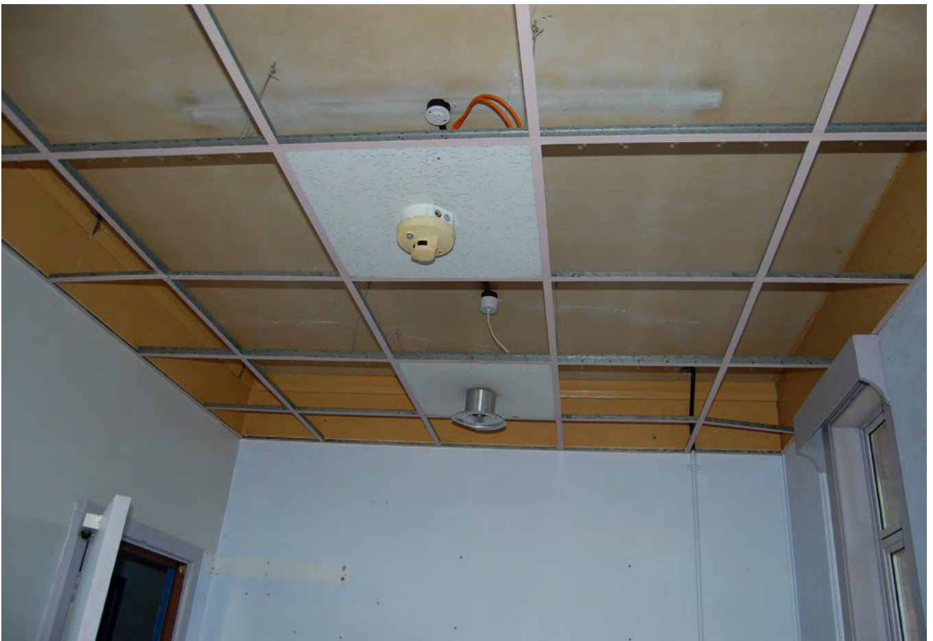
Plate 485.16 Ceiling staining showing the previous light fitting
