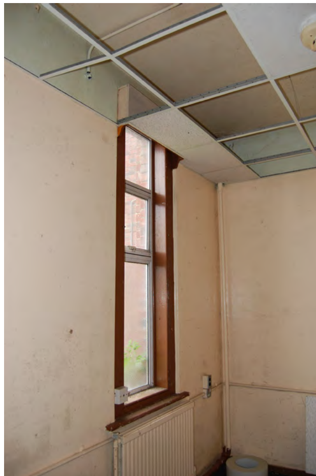
Plate 485.14 The suspended ceiling obscuring a ground floor window pelmet
