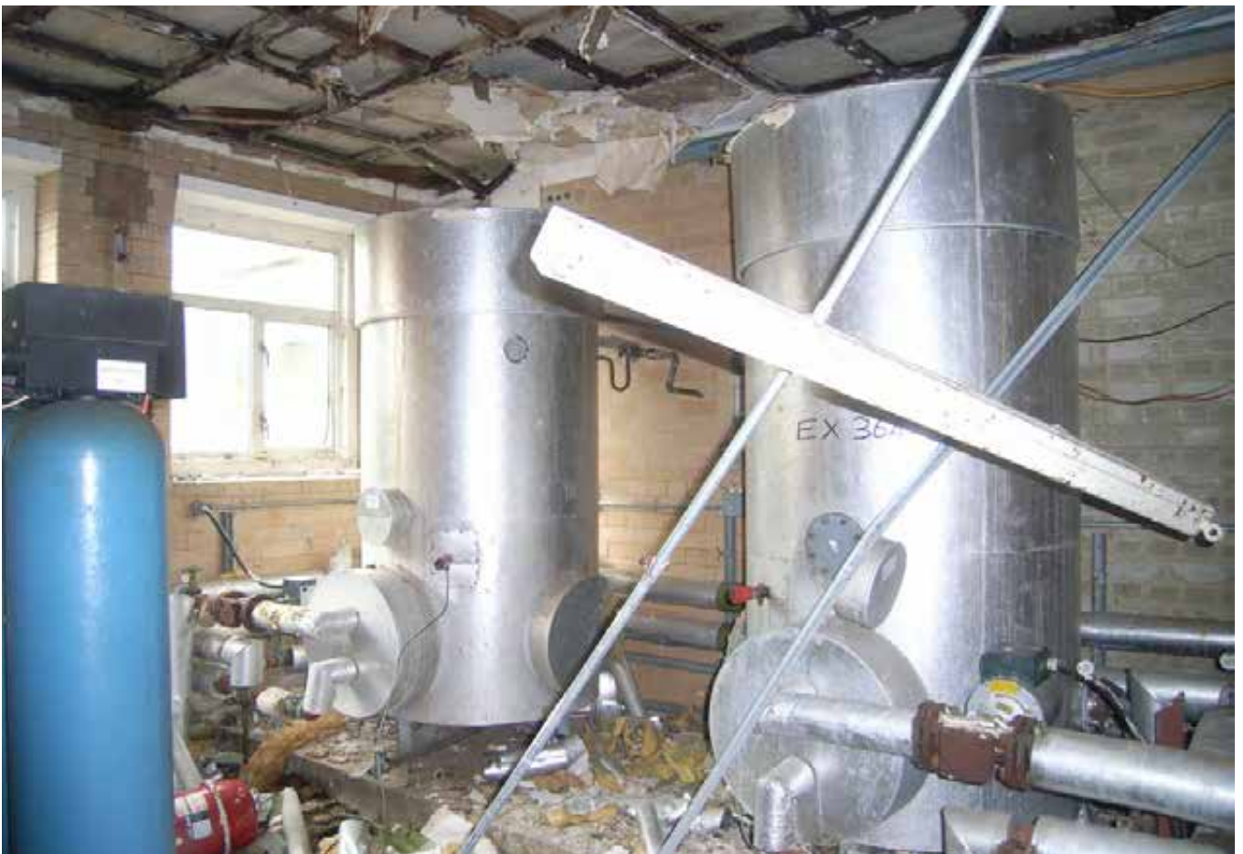
Plate 488.30 The calorifier room
