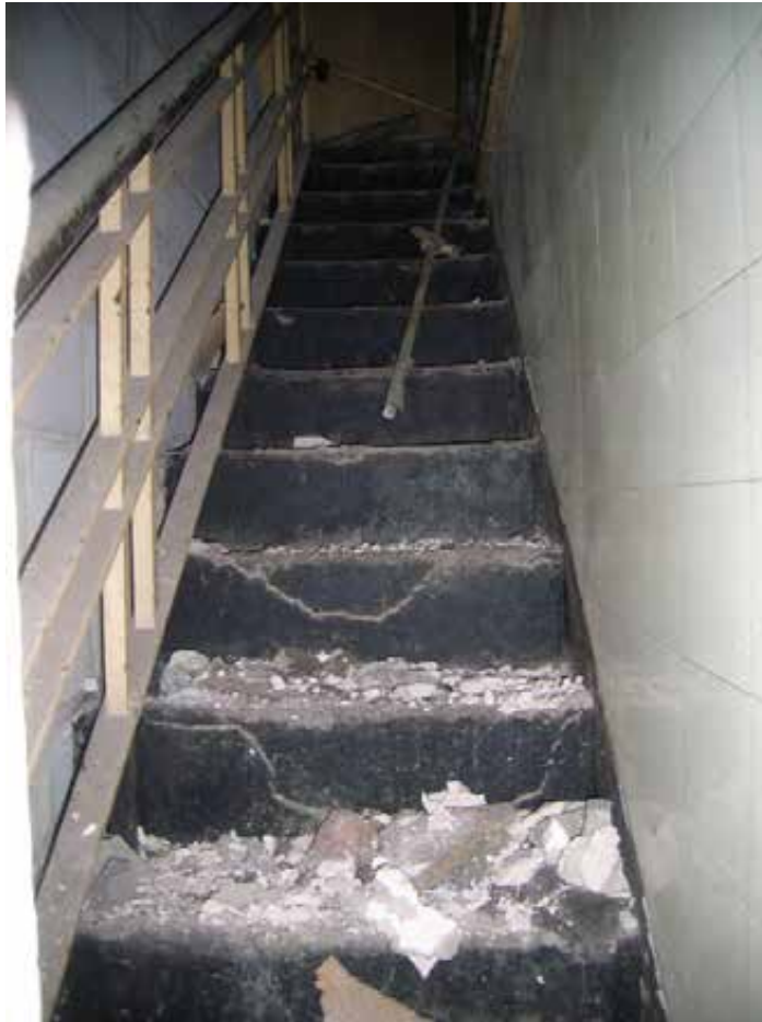
Plate 488.29 The blocked in staircase
