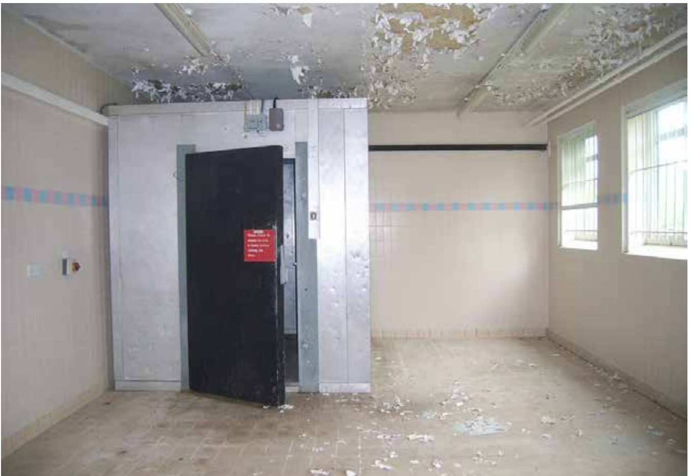
Plate 488.26 A walk-in refrigerator in the food storage area
