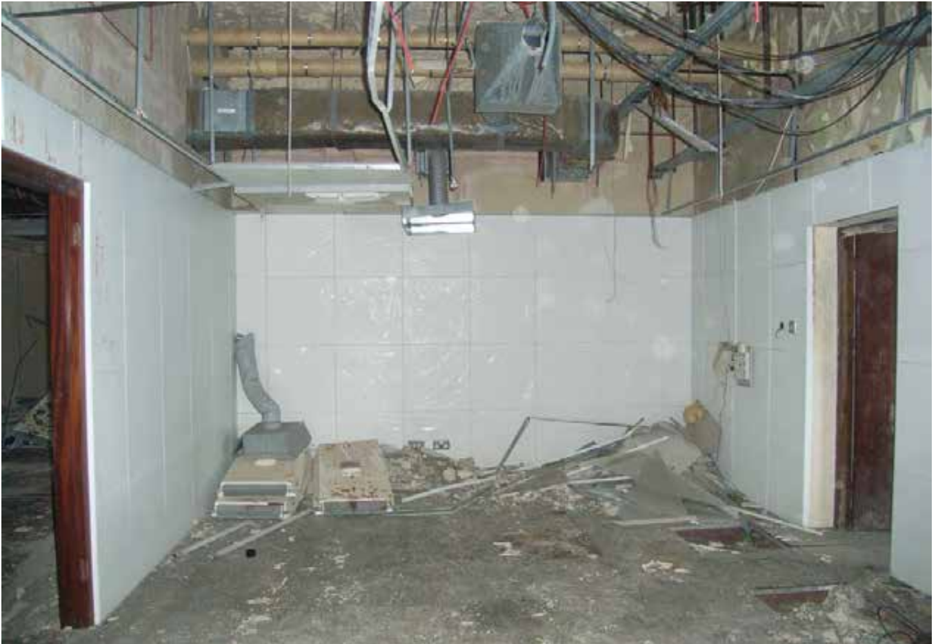
Plate 488.47 The server room
