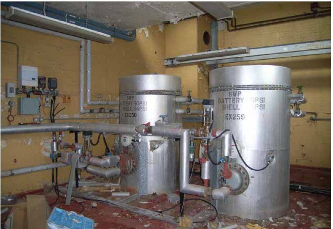
Plate 488.32 The boiler room
