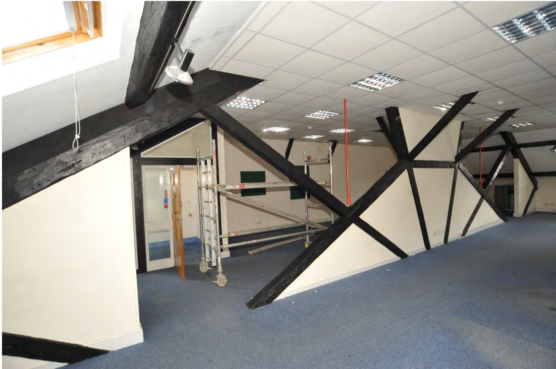
Pl.9: The exposed section of the westernmost truss, viewed from the second floor.
