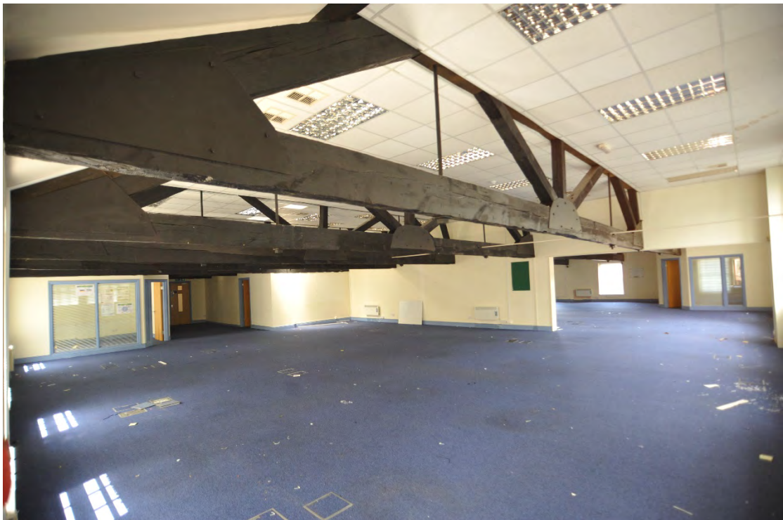
Pl.10: Some of the trusses visible at first-floor level; the tie-beams are in two sections.
