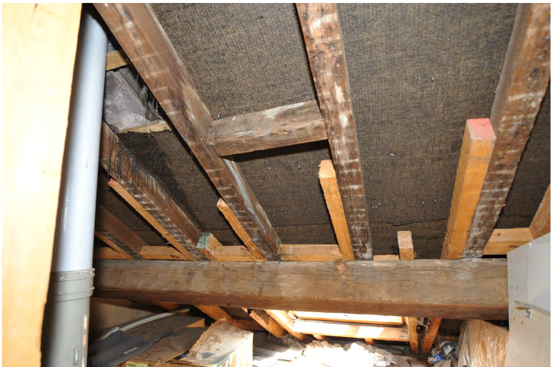
Pl.12: Evidence of lath-and-plaster in the roof space as well as trimmers between rafters and recently inserted rafters.
