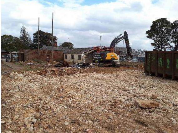
19.09.18 – View southeast from centre of northern boundary – demolition of Building 100 in progress.
