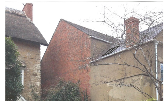
Photograph showing location of new roof window to be installed into existing slated roof
