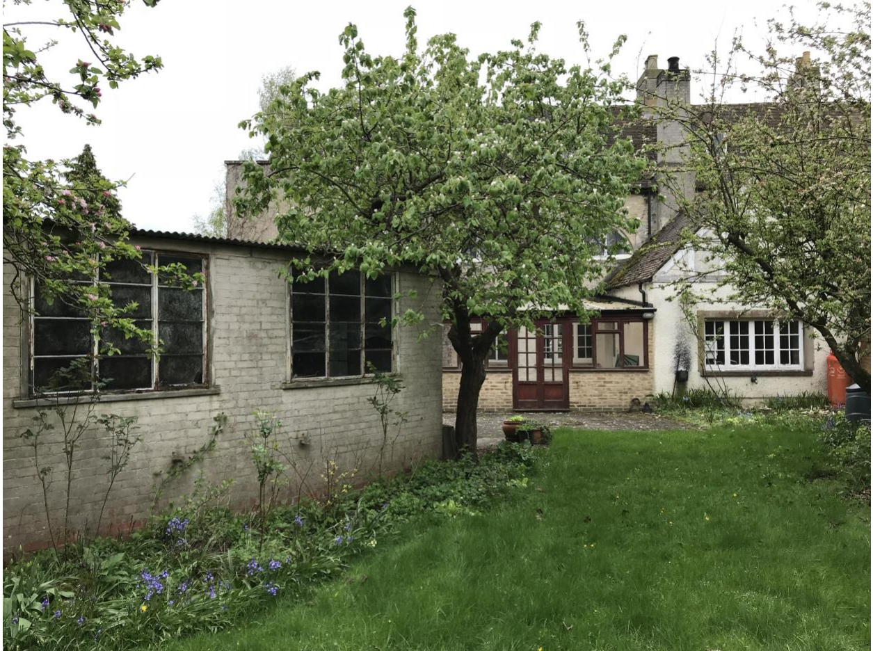
Existing flue location noted by extensive flue gas residue/marking to left of kitchen window
