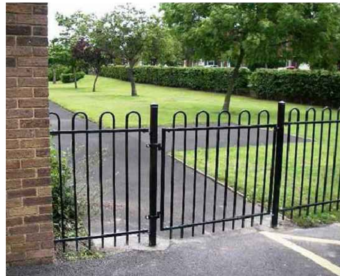
Similar typical bow top fencing
