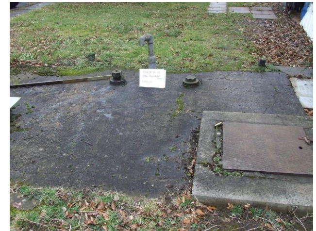
Photo 10 (right) showing tanks UGNSA 34 and 35.
