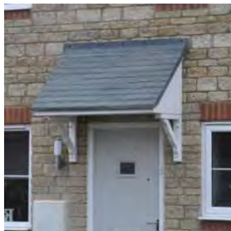
Unsuccessful example of plastic faux-tile porch, Banbury
