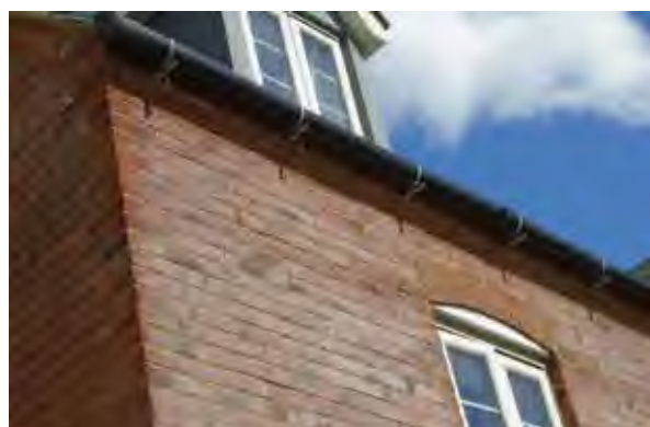
Guttering, South West Bicester
