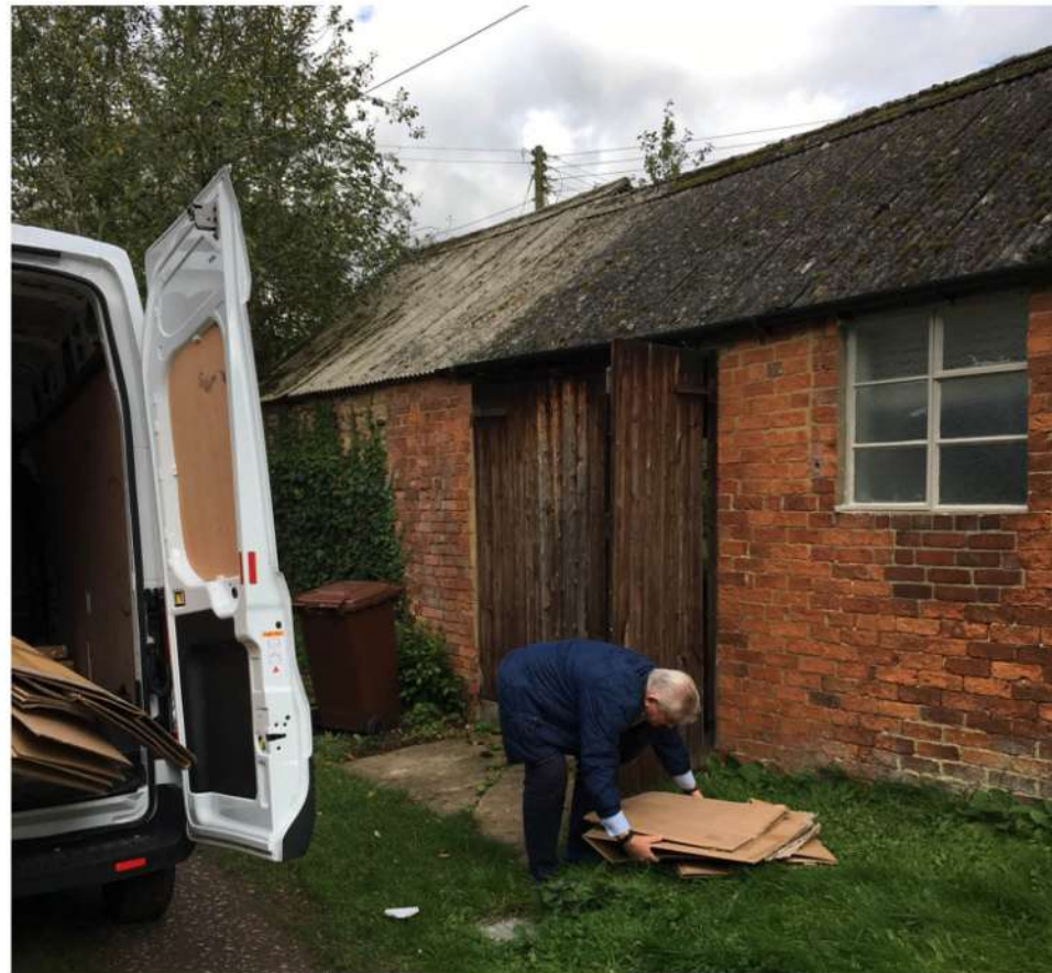
Existing Side Elevation of ancillary buildings: Garage door and metal frame window.
