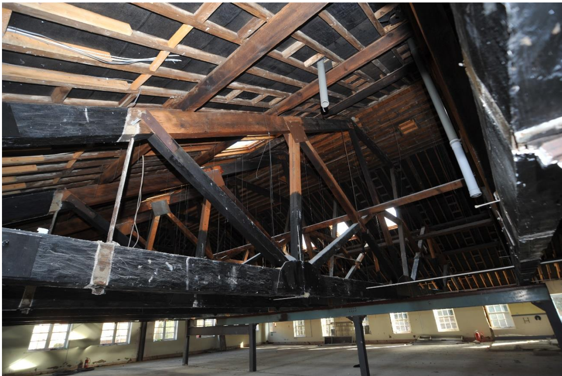
Pl.10: Some of the trusses exposed recently; the tie-beams are in two sections and the vertical studs are recent additions.
