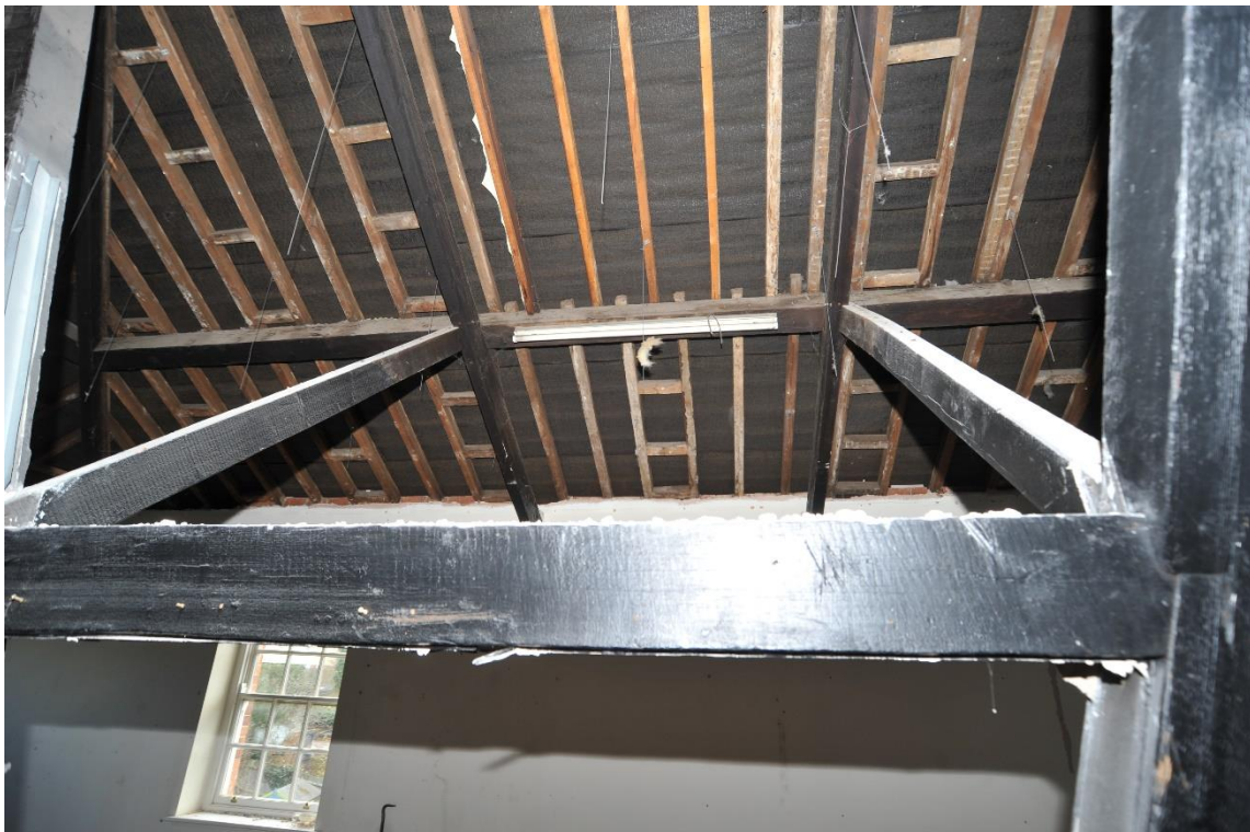
Pl.12: Evidence of lath-and-plaster in the roof space as well as trimmers between rafters indicating an original rooflight position and recently inserted rafters.
