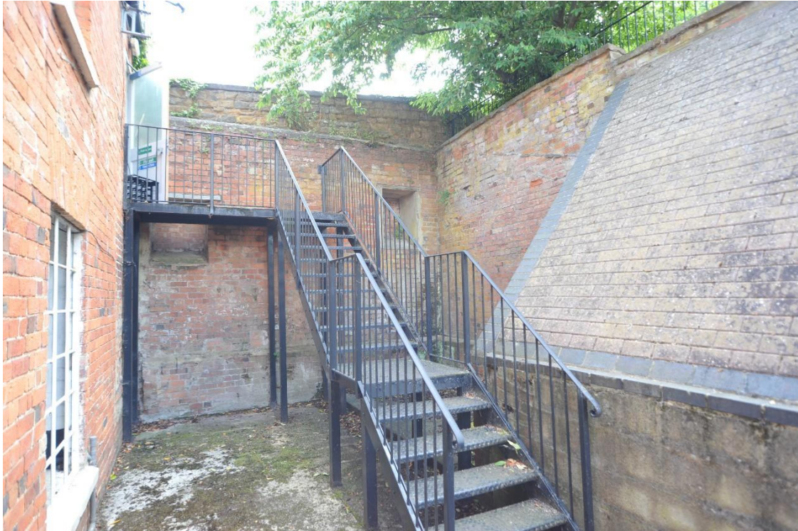
Pl.18: The eastern end of the rear yard with the brick wall and revetment of the terrace to the right. The area beyond the sloping section was once infilled with a building.
