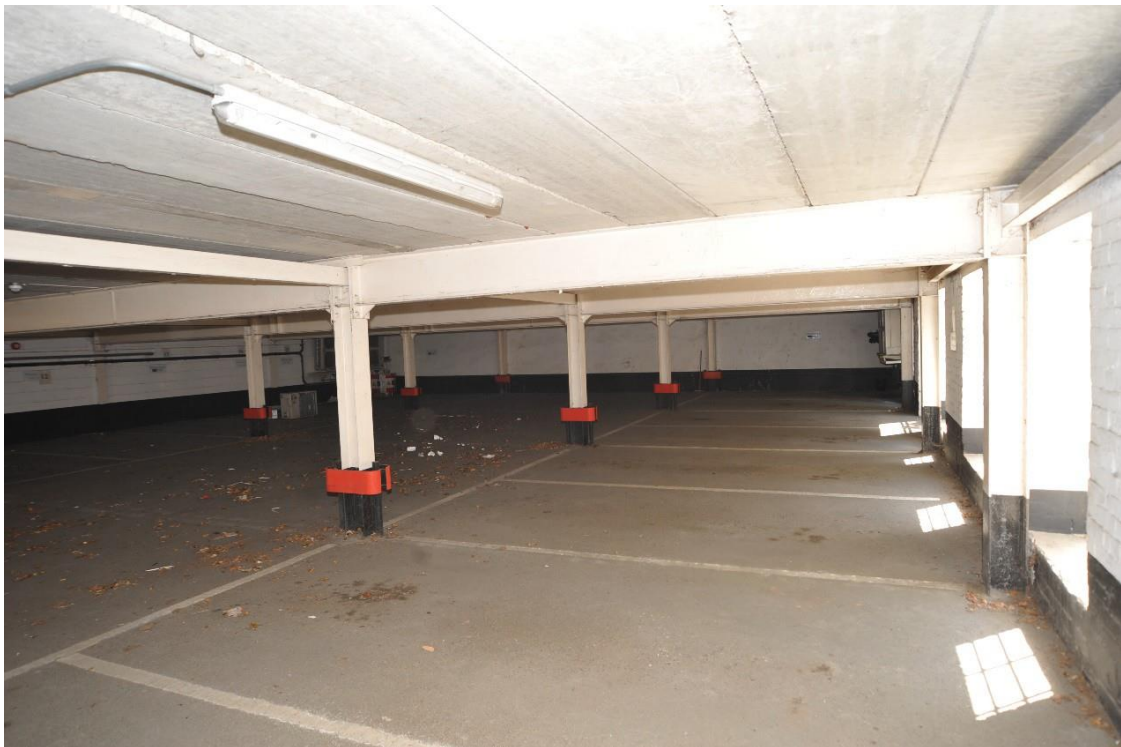
Pl.14: The bulk of the ground floor of the building is a covered car park; note the RSJ stanchions and concrete first floor, presumably dating to the engineering works phase.
