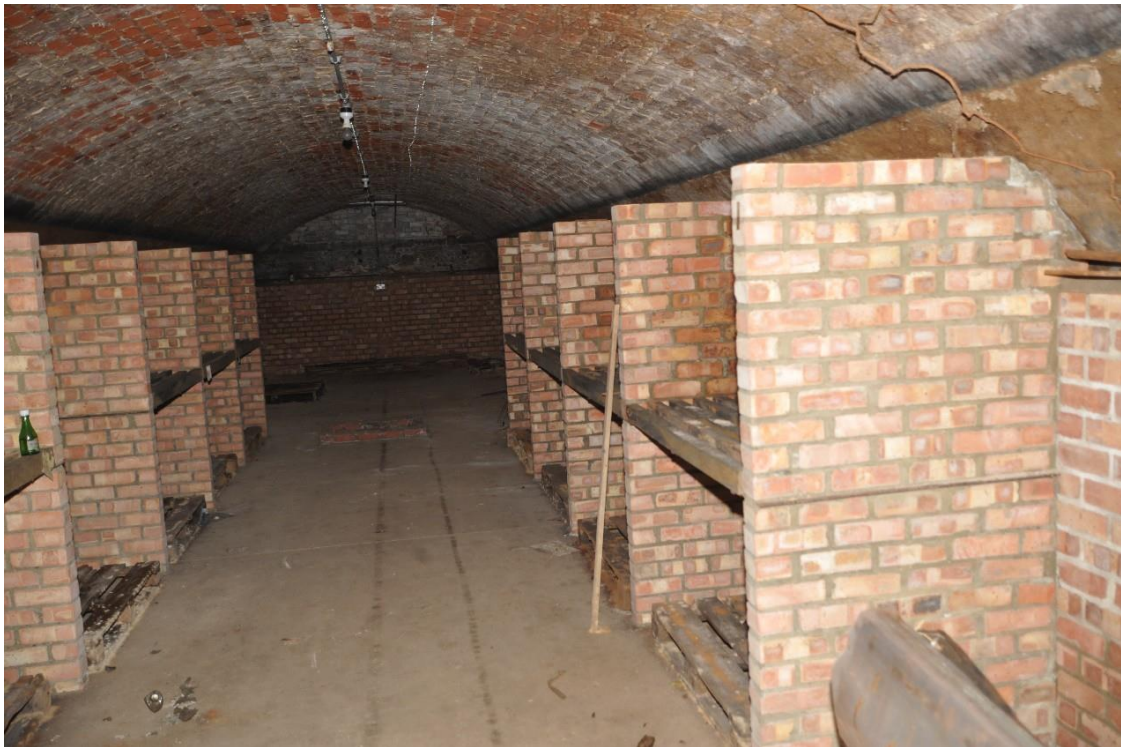
Pl.19: Below the terrace; the brick walls of the shelving is quite modern.
