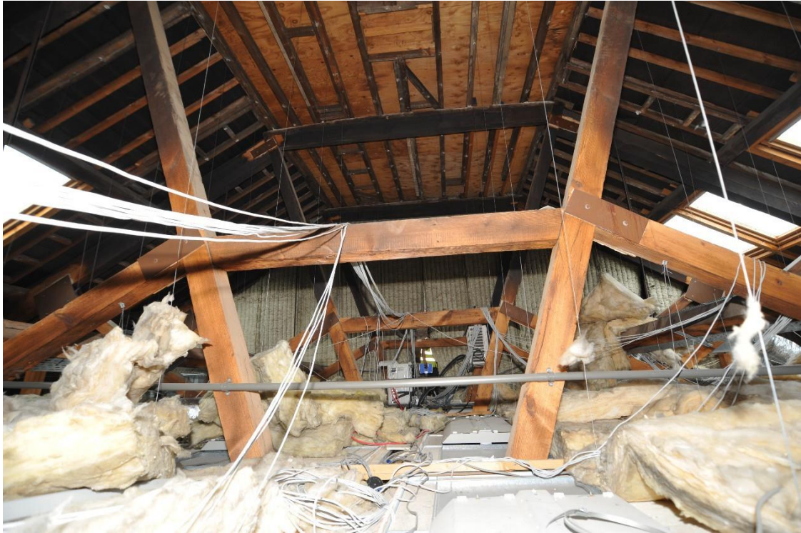
Pl.11: The tops of trusses visible above the ceiling in the main body of the building.
