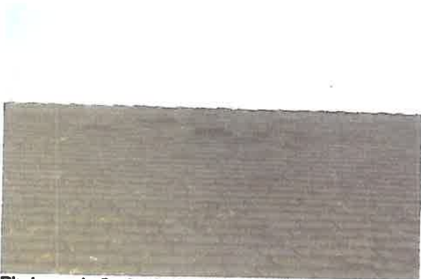
Photograph 3. A photograph showing some of the lifted wooden shingles.
