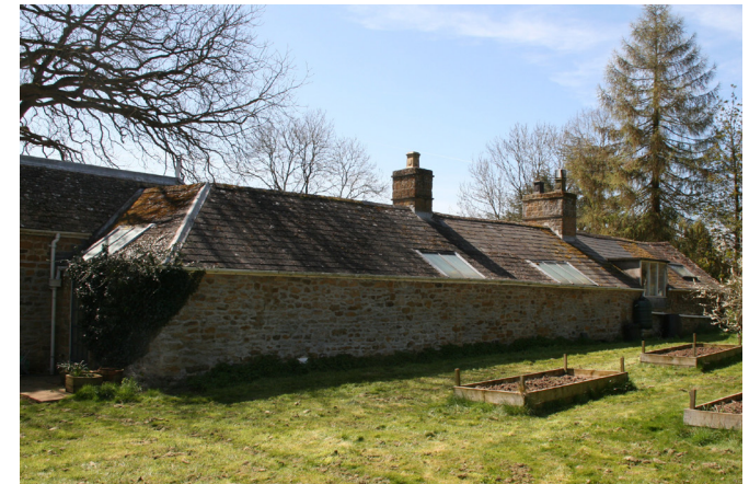
Rear elevation with rooflights in poor condition
