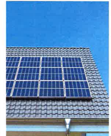
Energy created onsite - including through photovoltaic panels
