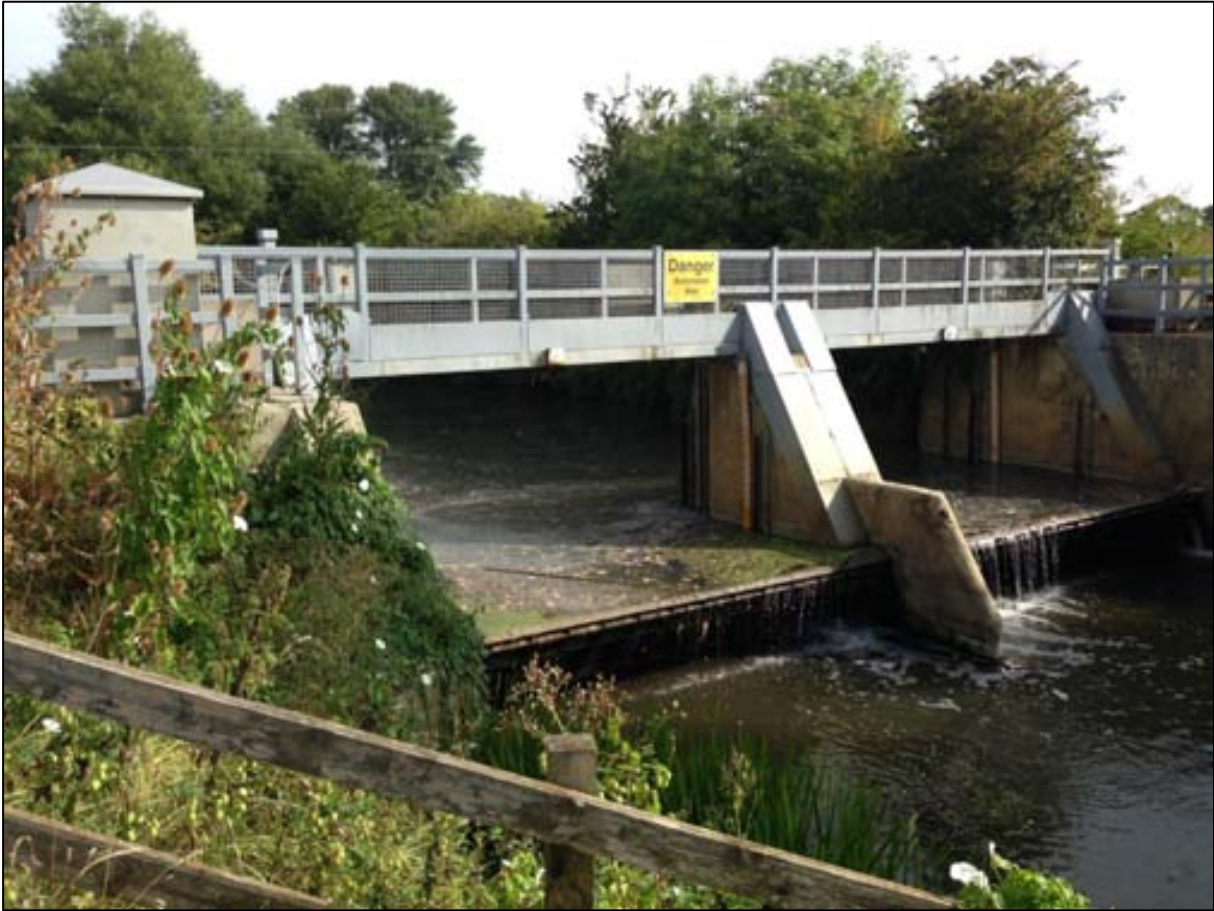
Figure 8 – Automated Weir at Islip
