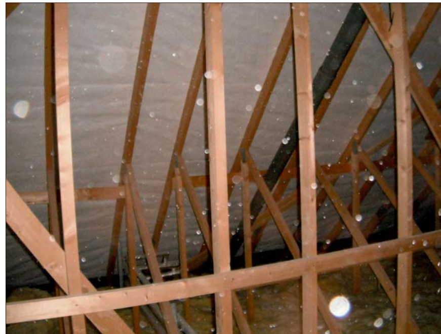
Photograph 2: Showing the cluttered attic space above the hotel.
