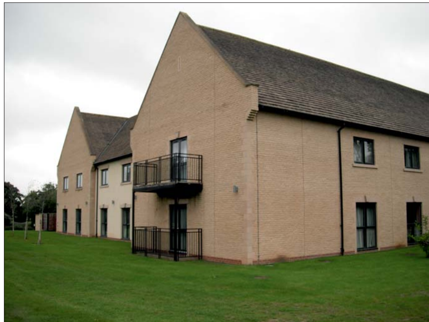
Photograph 1: Showing the rear and side elevation of the existing wing of the hotel and well-maintained amenity grassland.
