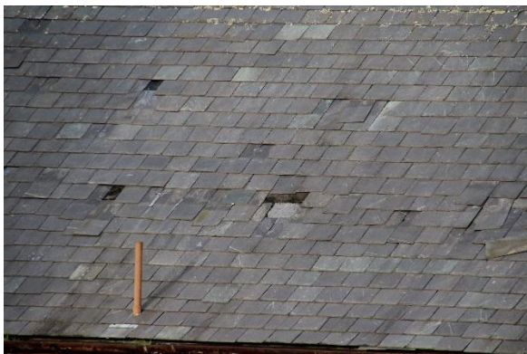
3. Slipped and missing tiles on Building 485
