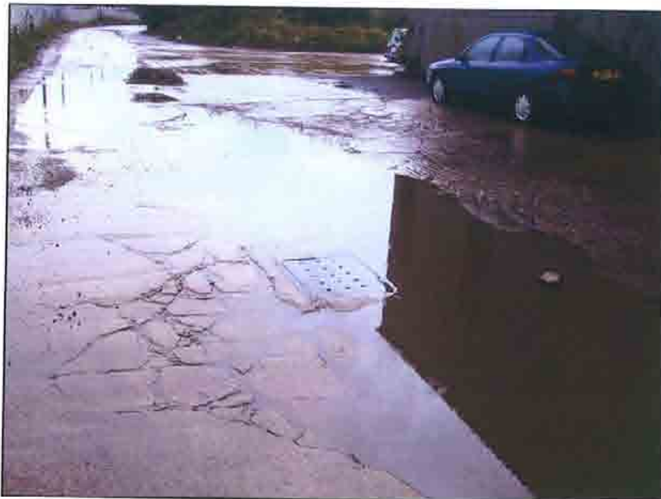
Plate 10: Collapsed drain outside Friswell Blackbushe.
