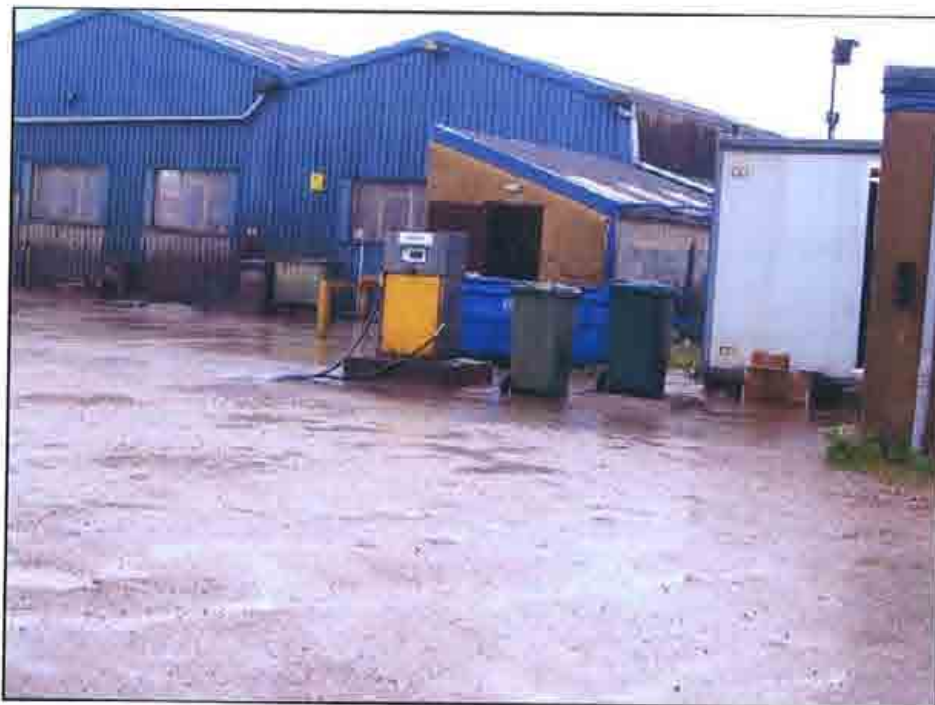
Plate 4: Diesel pumps in Grundon compound.
