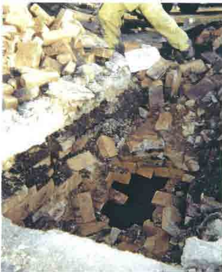
TP14 – Underground cavity
