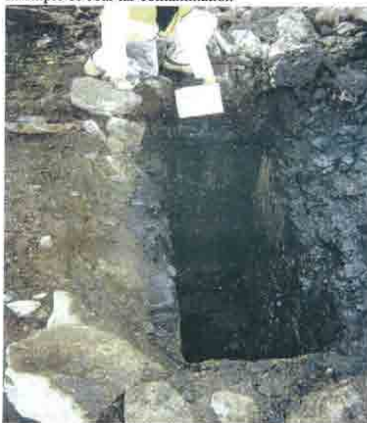
Tp08 – Coal tar contamination
