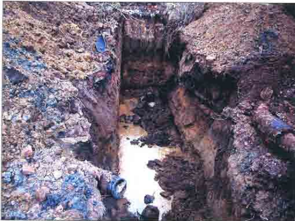
Plate 11: Underground pipework and contaminated groundwater - strong gas works odour noted
