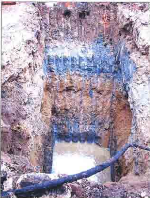
Plate 10: Alluvial sand and gravel beneath concrete pad - Strong gas works odour noted
