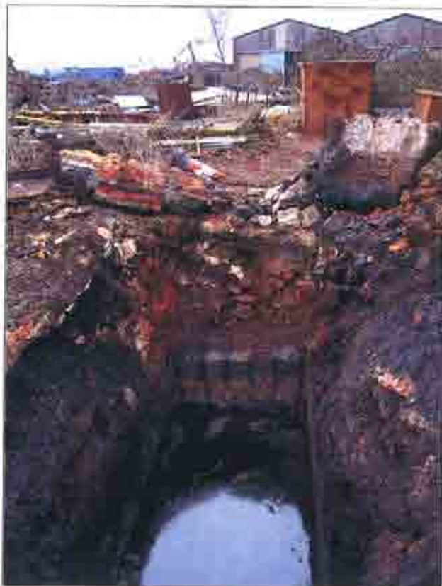
Plate 13: Free product encountered within made ground and alluvium
