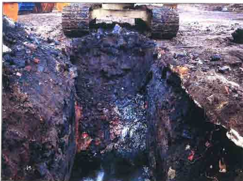
Plate 12: Significant inflow of tarry residues through north face of trial pit
