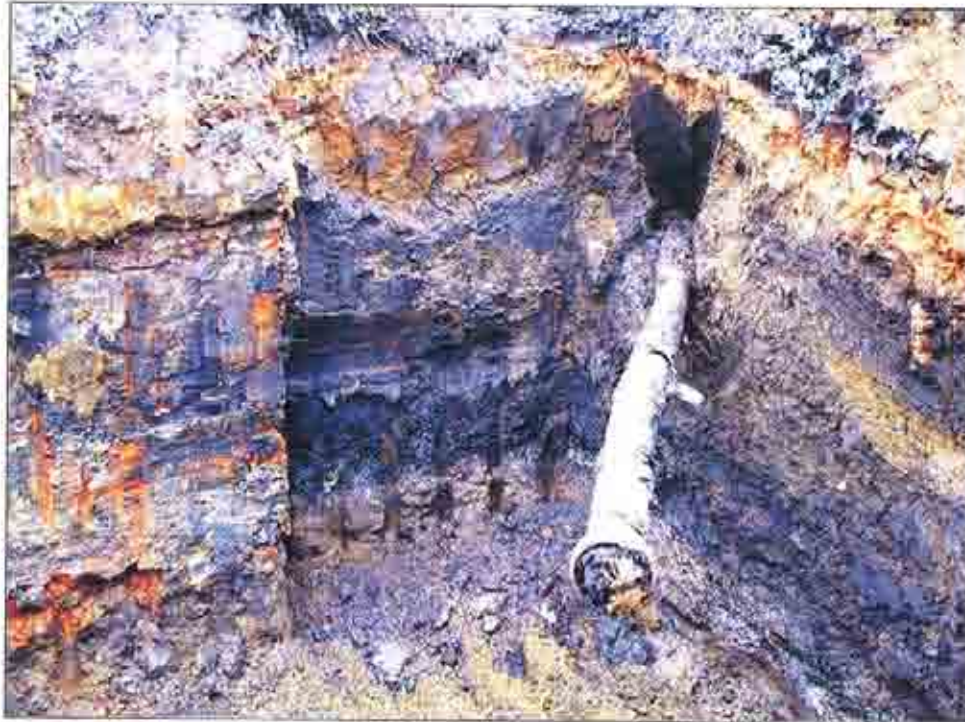
Plate 21: Western wall of Chamber 3 with 250mm Ø iron pipe at 1.2m bgl
