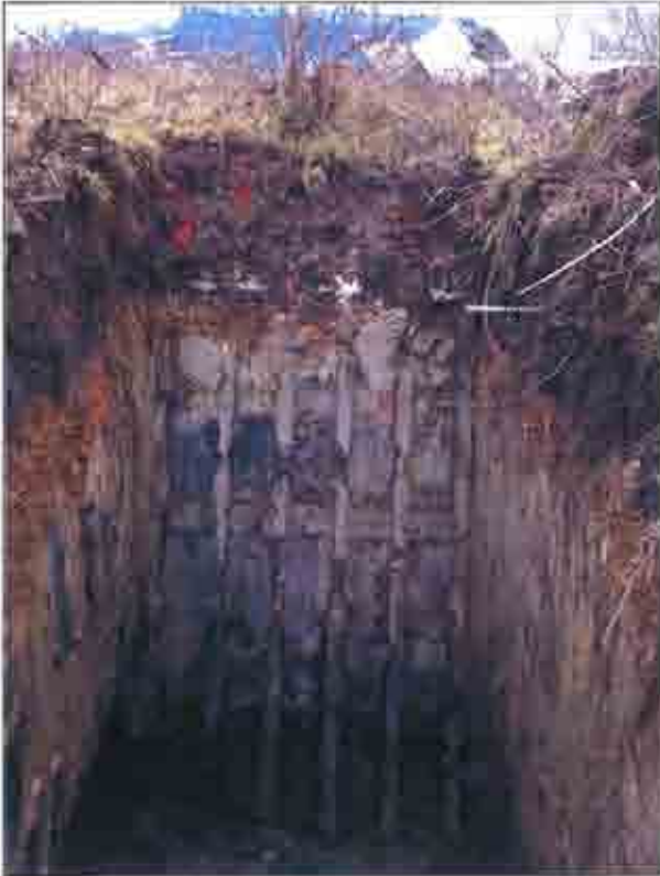
Plate 1: North western face of trial pit - upper sequence of made ground with contaminated alluvium beneath
