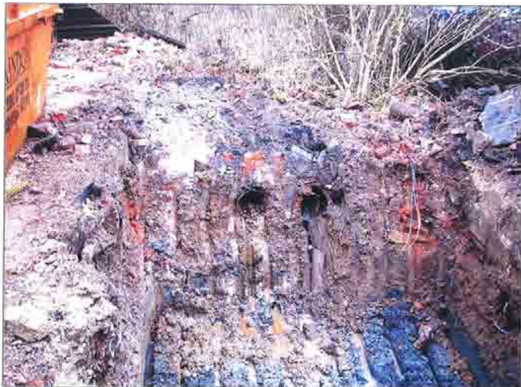
Plate 8: 2 x 250mm Ø iron pipework - Strong gas works odour noted
