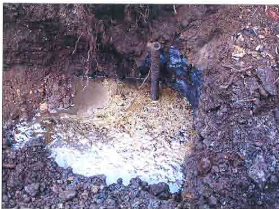
Plate 30: Contaminated water rising to surface from redundant pipework on the northern face of trial trench (noxious ammonia odour)
