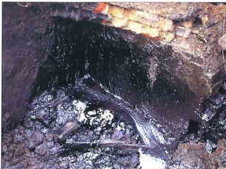
Plate 18: Vaulted roof of Chamber 2 with significant volume of tarry residues
