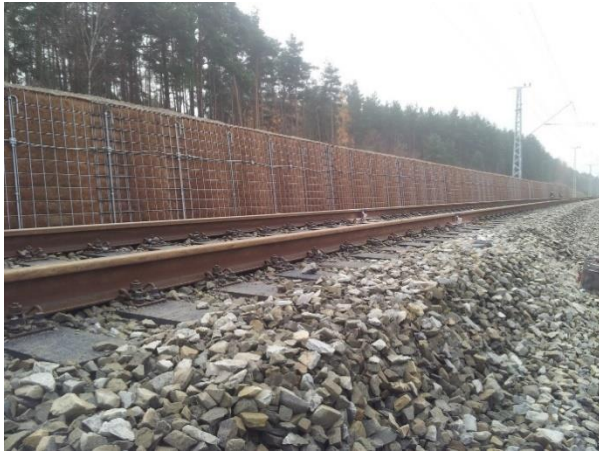
This photo shows a new installation alongside a railway line somewhere in the Netherlands
