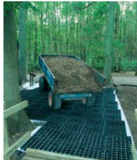
Glynebourne Wood. Pedestrian path to recreational wood and built using a CellWeb™ foundation which was covered with DuoBlock and then filled with woodchip to create a porous surface.
