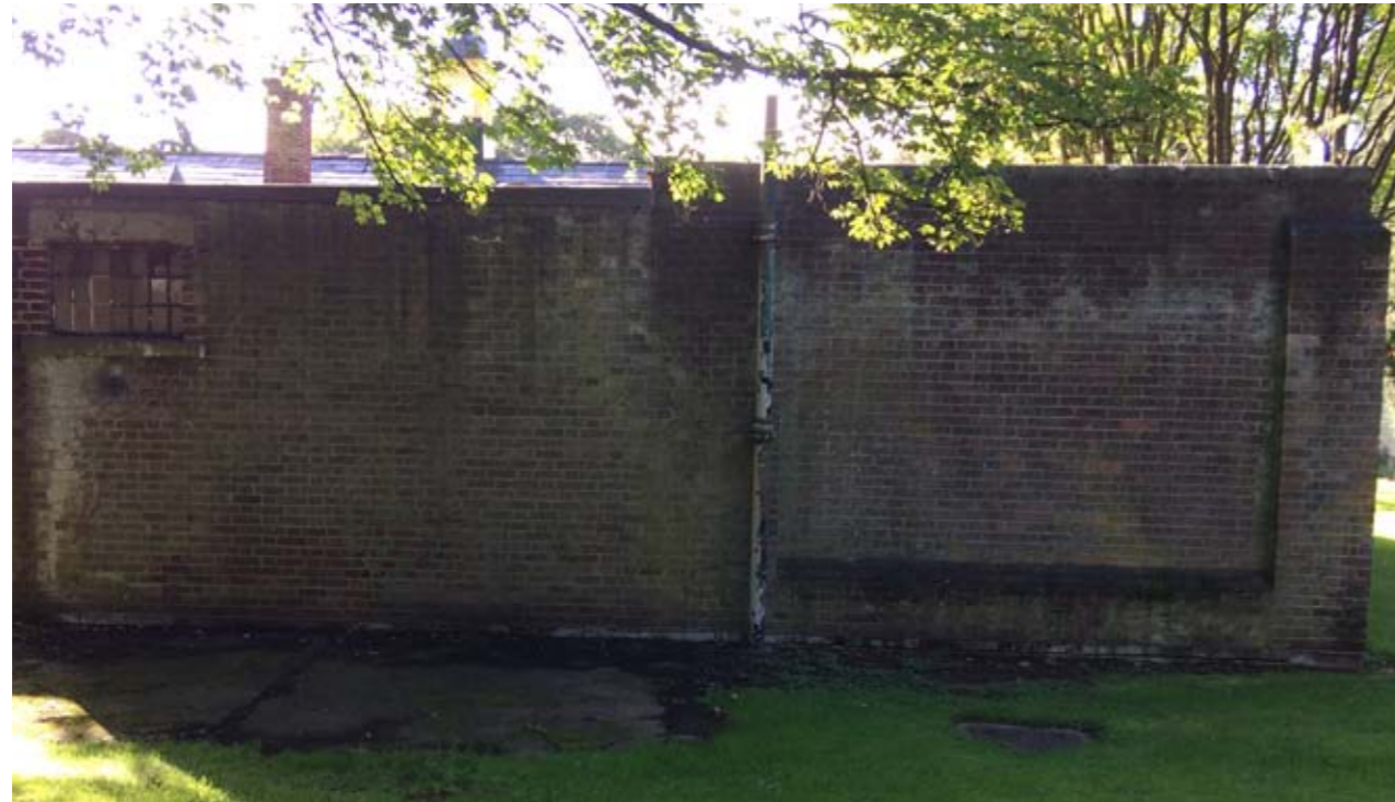
Fig 9. Side view showing the fortress like condition of the existing building, and use of red brick construction.
