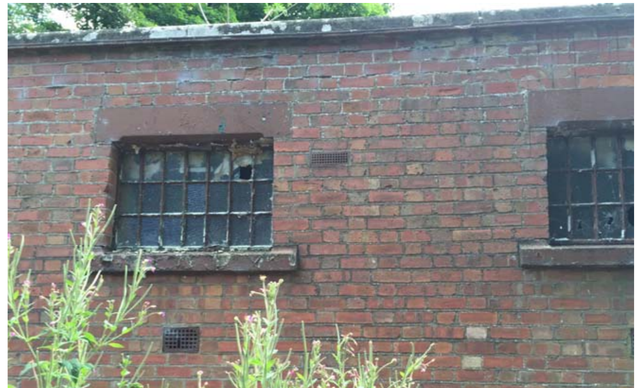
Fig 8. Example of existing high level prison windows to the side of the building.
