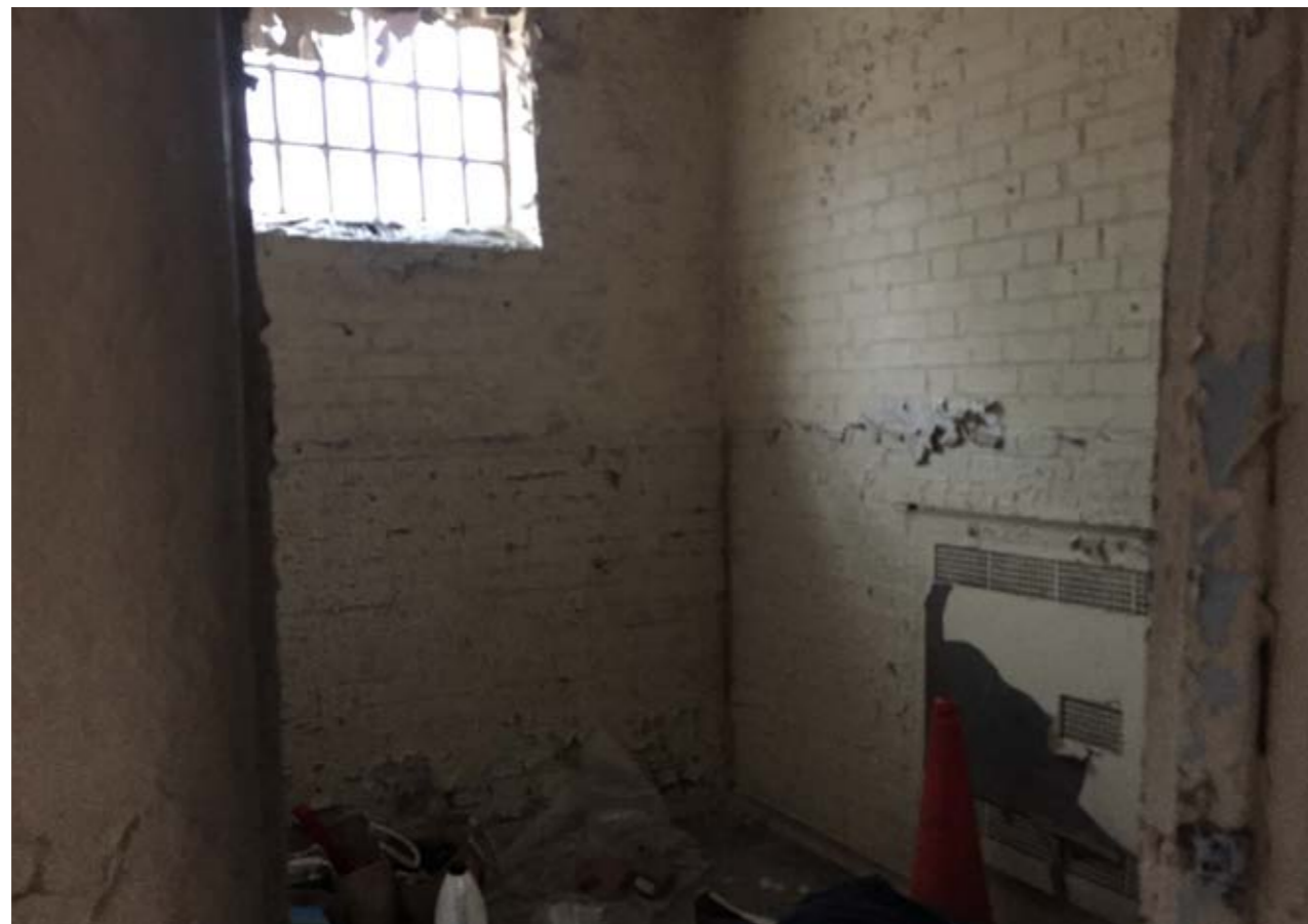
Fig 10. Internal view of the prison cells, showing the poor condition of the internal fabric in need of improvement.
