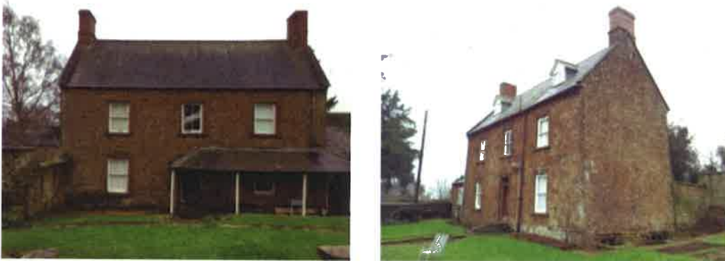
Plates 1 and 2. Yew tree House: north elevation showing the main house and canopy from the rear garden (left), and south-east corner showing the east gable wall with cellar windows just visible (right); the single-storey extension is proposed on the east gable wall (right).
