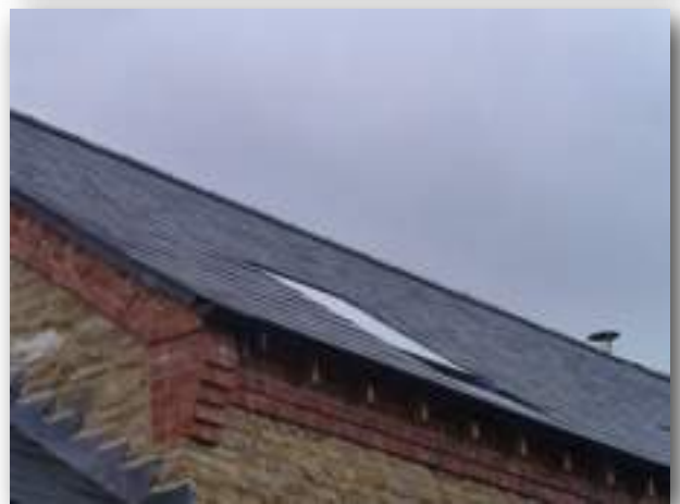
The above photographs show a recently installed “Neo” rooflight flush fitting within a slate roof and clearly shows how simple the glass panel looks
