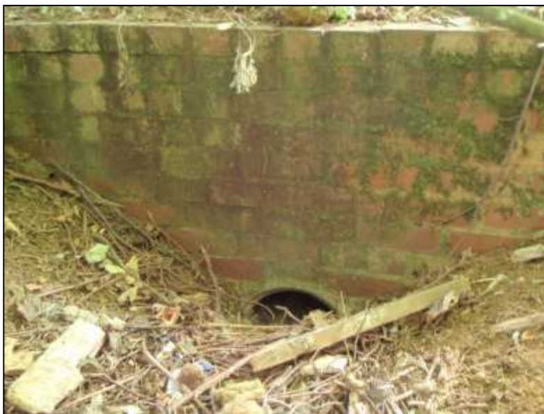
Photo 1. Brick Headwall at Culvert Inlet on Southern Site Boundary (Field Drainage Ditch).
