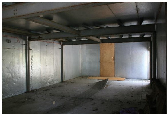
4. Interior of a refrigeration unit
