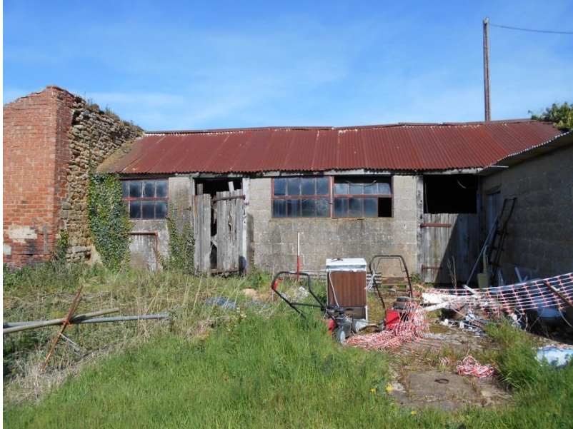
Fig 13: Building 7 of the 1970s, looking north; scale 1m. To the left is the ruinous Building 6 and to the right Building 8.
