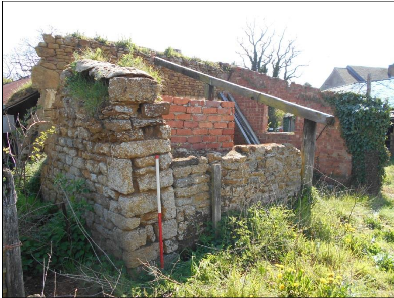
Fig 12: The ruinous Building 6, looking south-east. Sheep-dip out of view at bottom left; scale 1m
