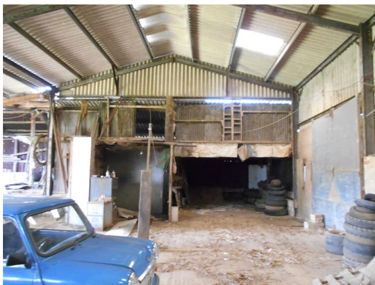
Fig 16: The interior of Building 10, a post-1974 steel-frame shed, looking west; Building 9 to left rear
