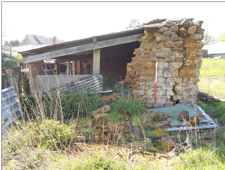
Fig 11: The northern half of Building 5, looking south, collapsed gable; scale 1m
