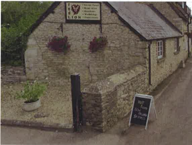
Rain Water Down Pipe discharging to road
