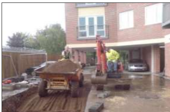
Structural soil image 1: Structural tree soil retains sufficient structure for tree roots to grow, even when compacted.
