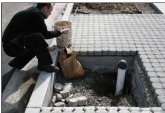
Soil cell image 3: The finished surfacing is profiled to leave the tree pit open, ready to be filled with good quality topsoil and the new tree.
