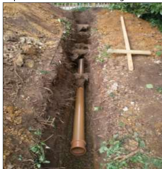
Services image 2: Continuous trenches dug by hand so that important roots can be retained (with the service ducting threaded beneath) is an effective means of minimising damage (note the ground protection boards with soil piled on top on the left).
