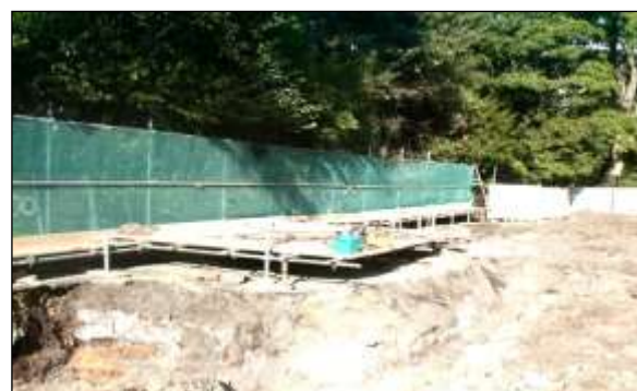
Ground protection image 4: A scaffold framework attached to the main scaffold fencing can be used to support either scaffold planks or plywood to create an elevated platform.
