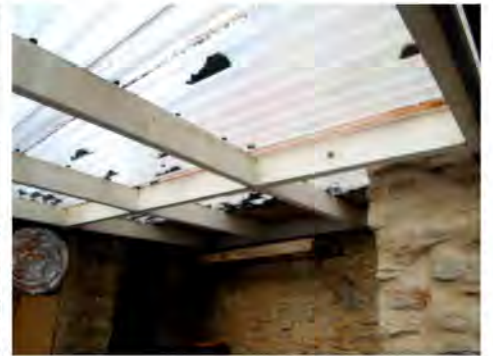
5.2 Canopy to be replaced
