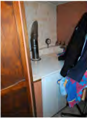
1.1 Boiler to be replaced
