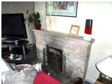
1.2 Fireplace to be replaced
