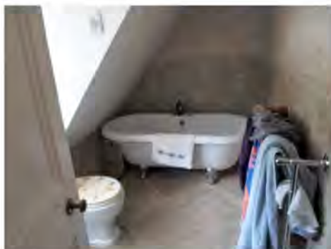
2.5 Bathroom 2 bath to be replaced
