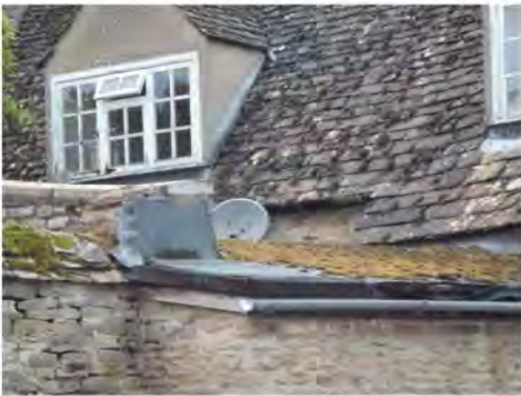
4.8 Satellite dish to be retained
