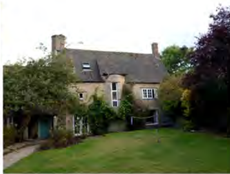
4.5 Rear slope to be re-tiled
