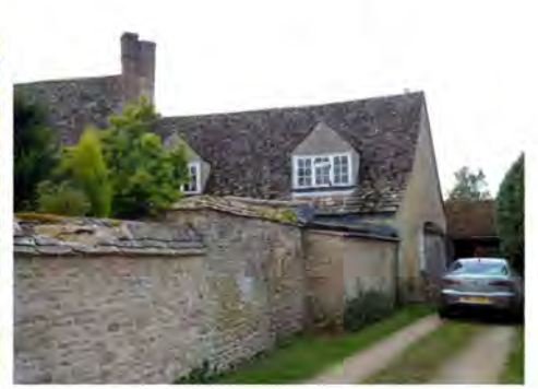
4.2 Felt roof to be re-covered
