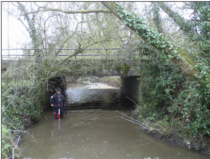
Figure 9 – Upstream Face of Langford Lane Road Bridge, Modelled as a Culvert Unit at ISIS node LB6
