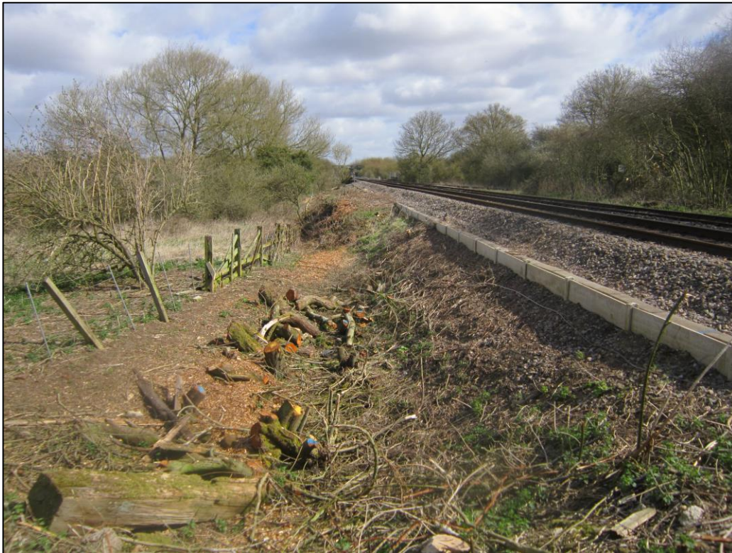
Figure 17 – Photograph of the Northern Surface Water Drainage Ditch to be Partially Filled, taken from within the ditch – Atkins, 2013.
