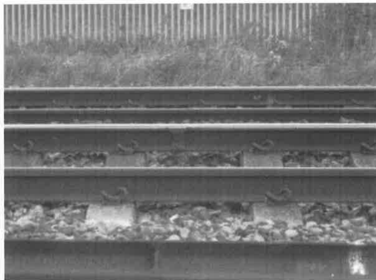
Photograph 11: DCL Line Up Main 6' rail 65m 501yards. L80 wide gap weld
