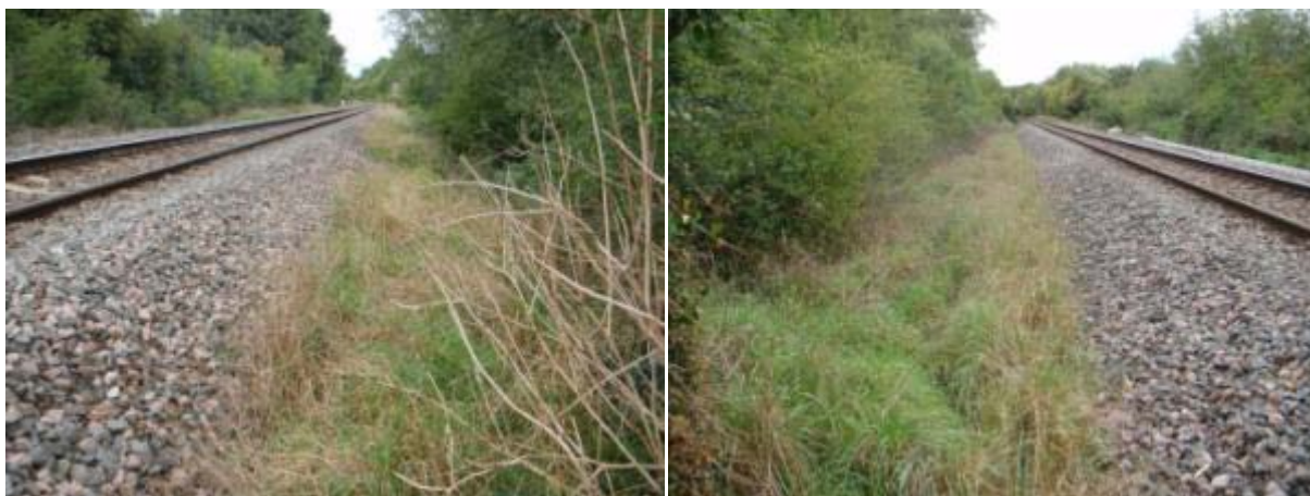
Photograph 6 and 7: Down Cess (left hand side facing Oxford) looking towards Islip (left) and Oxford (right) ballast shoulder and cess
