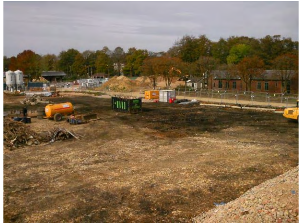
22.10.14 - Waste processing area in the north of the site, waste awaiting off-site disposal/recycling
