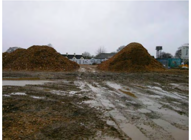
12.01.15 – Temporary stockpile of waste wood which has undergone processing (chipping) awaiting removal off-site
