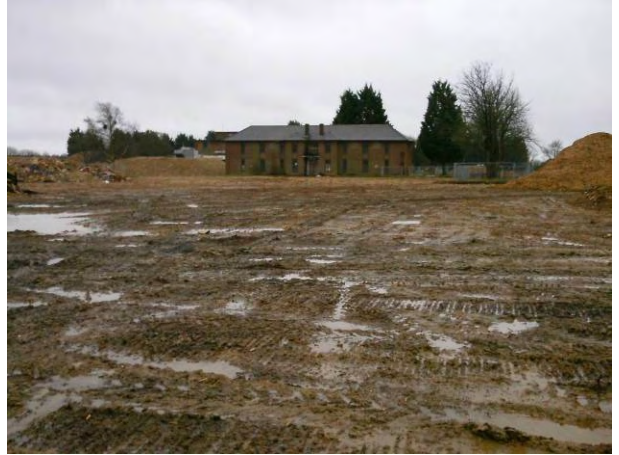
12.01.15 – Southern view down the centre of the site, northern face of building 465 visible.
