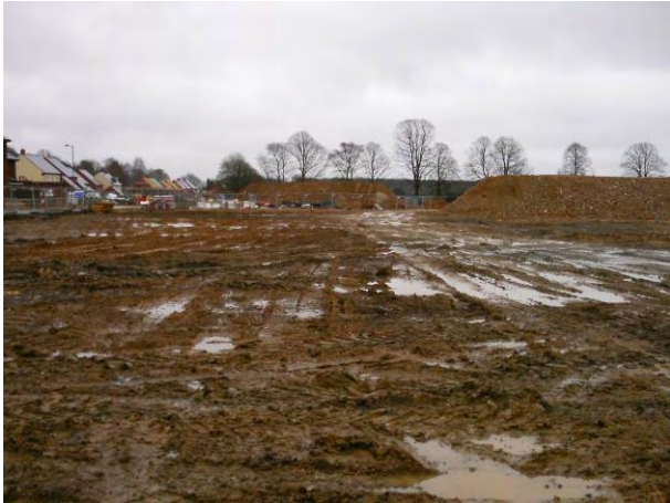
12.01.15 – Eastern view across the north of the site following completion of earthworks, D1B:Area 1 visible in the background
