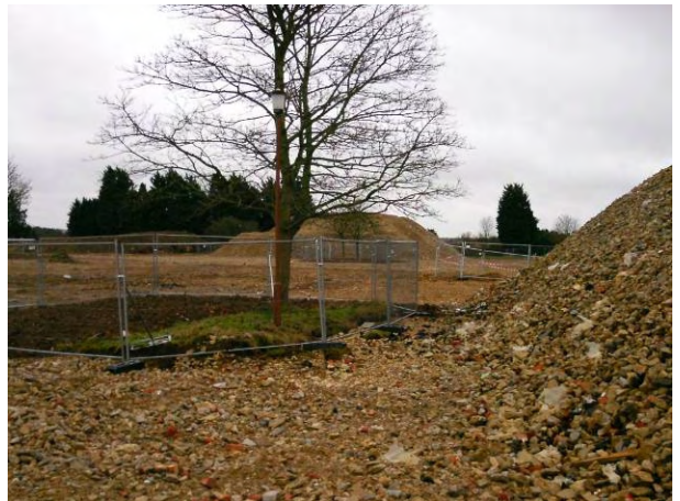
12.01.15 - Southern view from the centre of the site, stockpile Agg-SW visible in background
