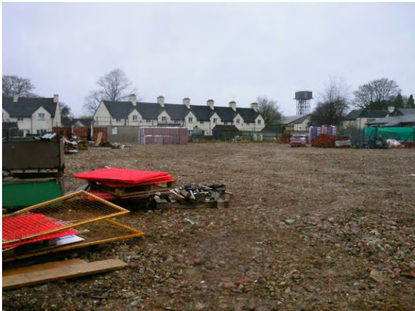
12.01.15 – North-west corner of the site being utilised as a brick store following completion of earthworks
