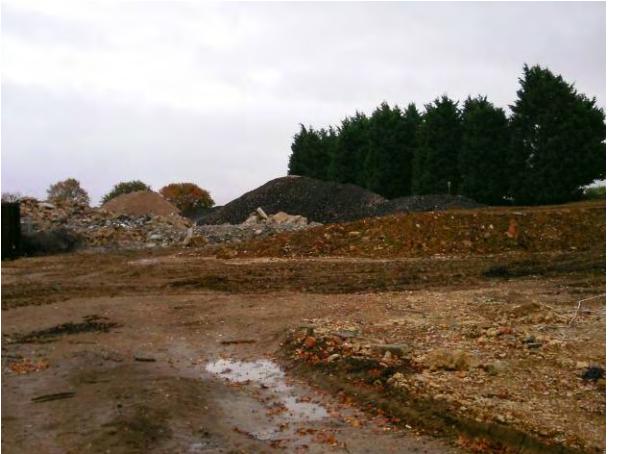
07.10.14 Stockpile storage area in the south with tarmac, subsoil and concrete awaiting processing
