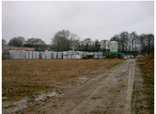
12.01.15 - North-west corner of the site being utilised as a brick store following completion of earthworks. Retained road which not remediated.
