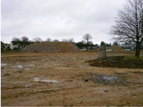
12.01.15 – Western view across the site following completion of earthworks, stockpile Agg-W visible in the background
