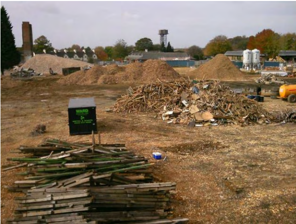
22.10.14 – Waste processing area in the north of the site, waste awaiting off-site disposal/recycling
