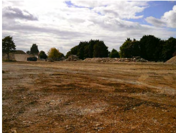
24.09.14 Removal of hard-standing exposed natural soils across the south-west of the site
