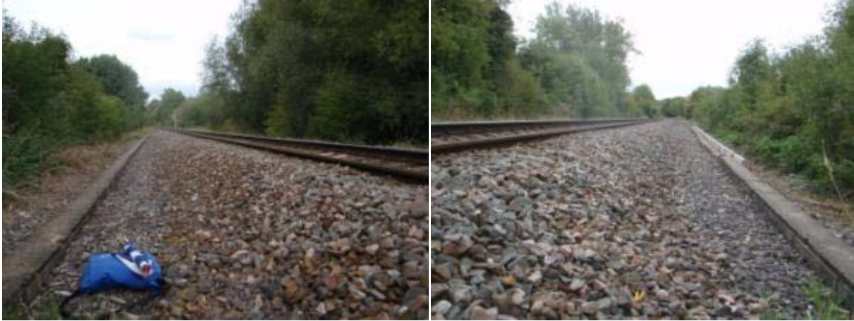
Photograph 4 and 5: Up Cess (right hand side facing Oxford) looking towards Islip (left) and Oxford (right) ballast shoulder and cess
