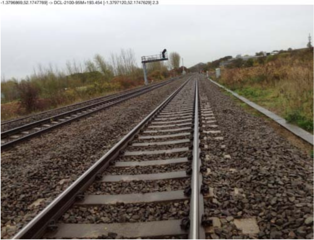
Photograph 13: DCL Down Line (looking towards oncoming trains) at 95m 9chain Looking towards Banbury
