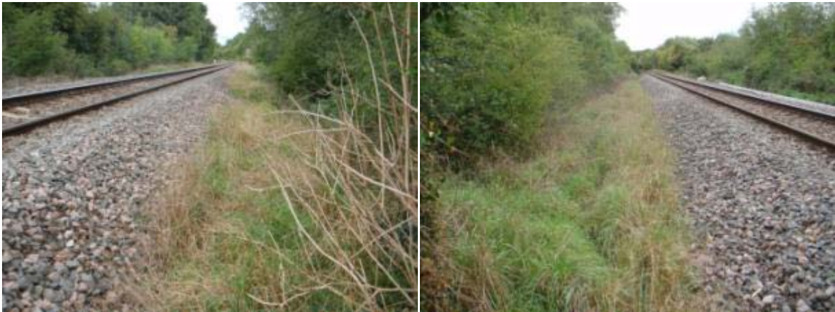
Photograph 6 and 7: Down Cess (left hand side facing Oxford) looking towards Islip (left) and Oxford (right) ballast shoulder and cess
