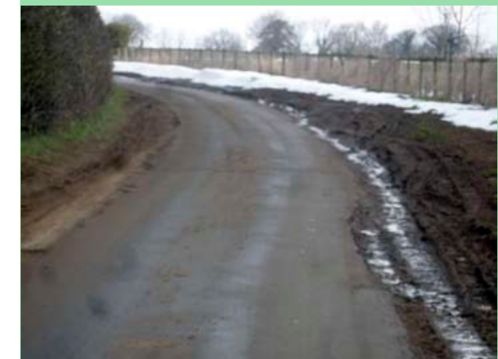
Significant erosion to Lane edges.
