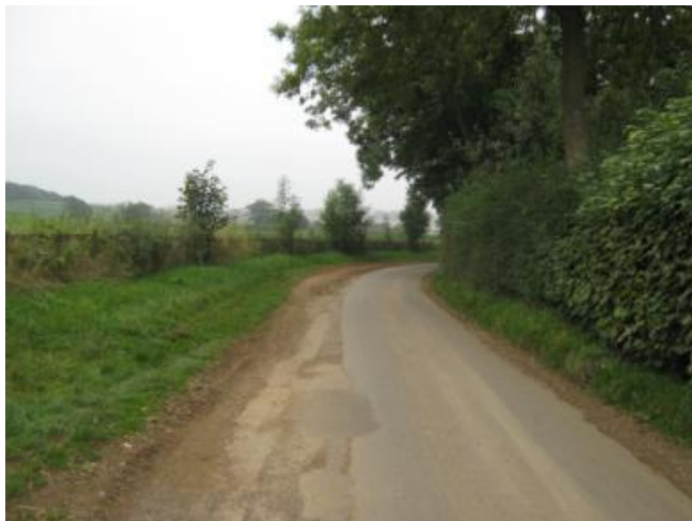
View of the damage in Grange Lane
